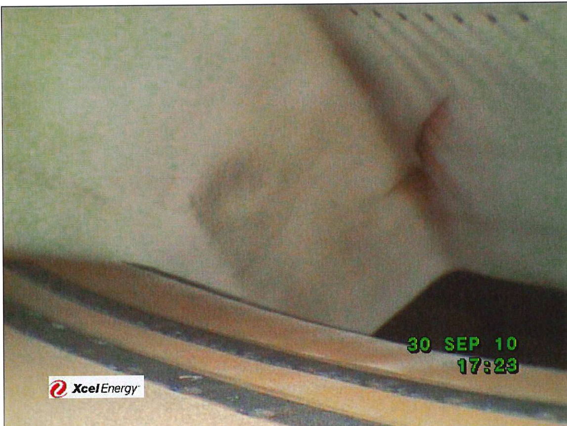
Burner #8 transition showing what appears to be a crack in the TBC coating. It does not appear to be a crack in the transition itself due to its orientation. This is not believed to be significant.
