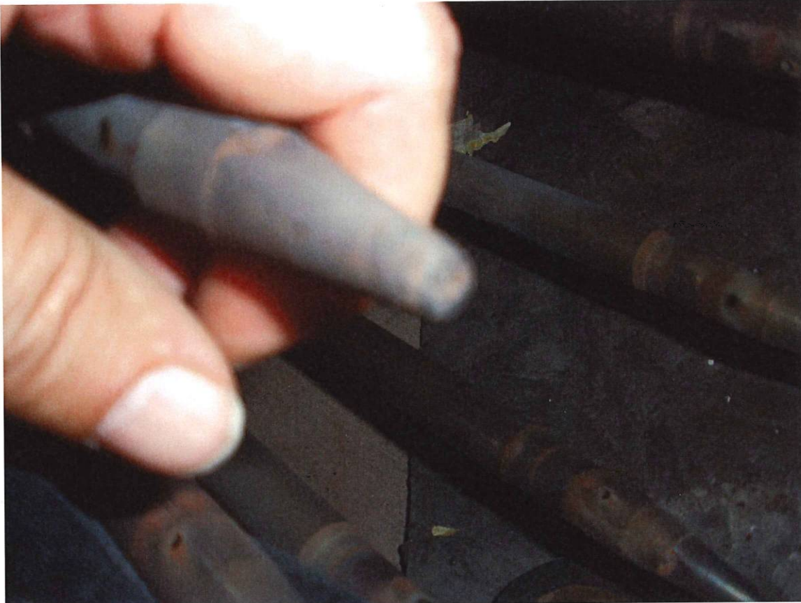
Blunt tip on one of the rocket tips. While not of major concern it does bear monitoring if the outage is indefinitely delayed (beyond fall 2011)
