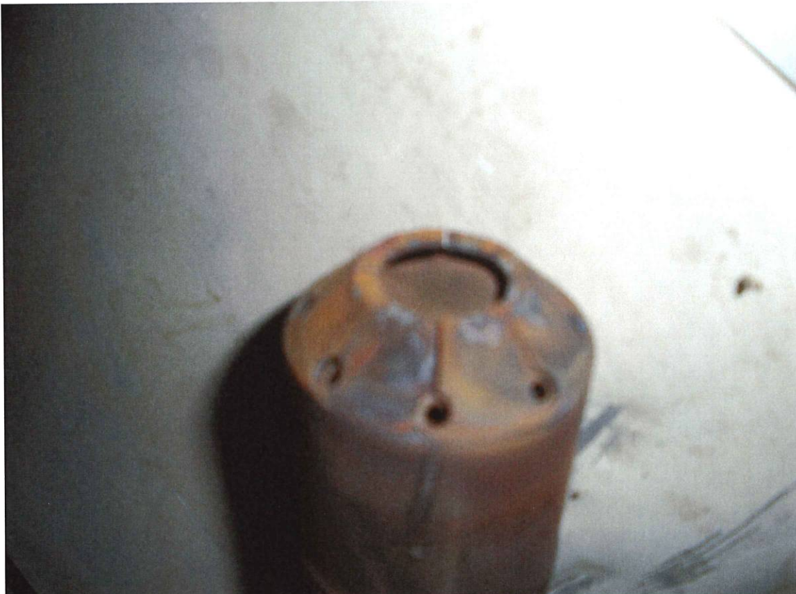
Burner #14 pilot nozzle tip. Note the discoloration on the tip, but this is fairly typical. No obvious signs of distress associated with the fretting shown above.
