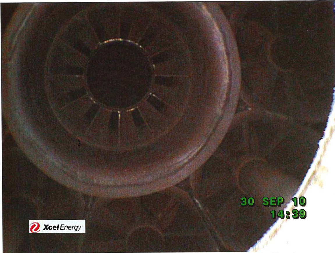
A slightly wider view of the pilot swirler on burner 3. No signs of any significant deterioration.
