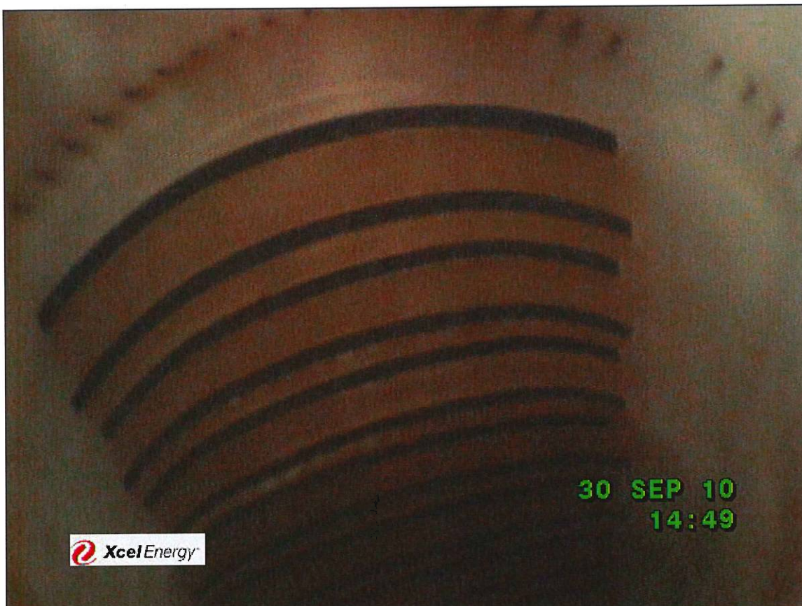
Borescope photo of the transition piece from burner #14. No signs of cracking, distortion, plugged cooling holes or other issues
