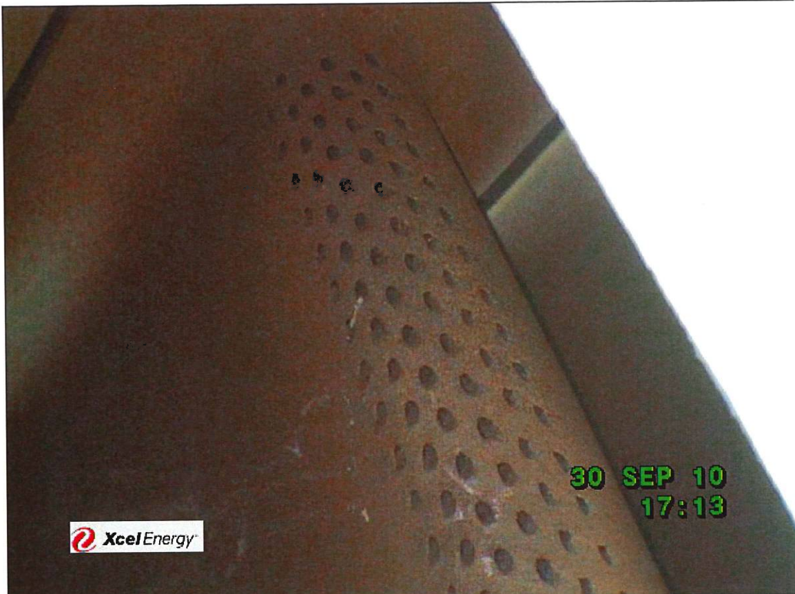
Row 1 vane at burner #8 No signs of cooling hole cracking or other signs of distress
