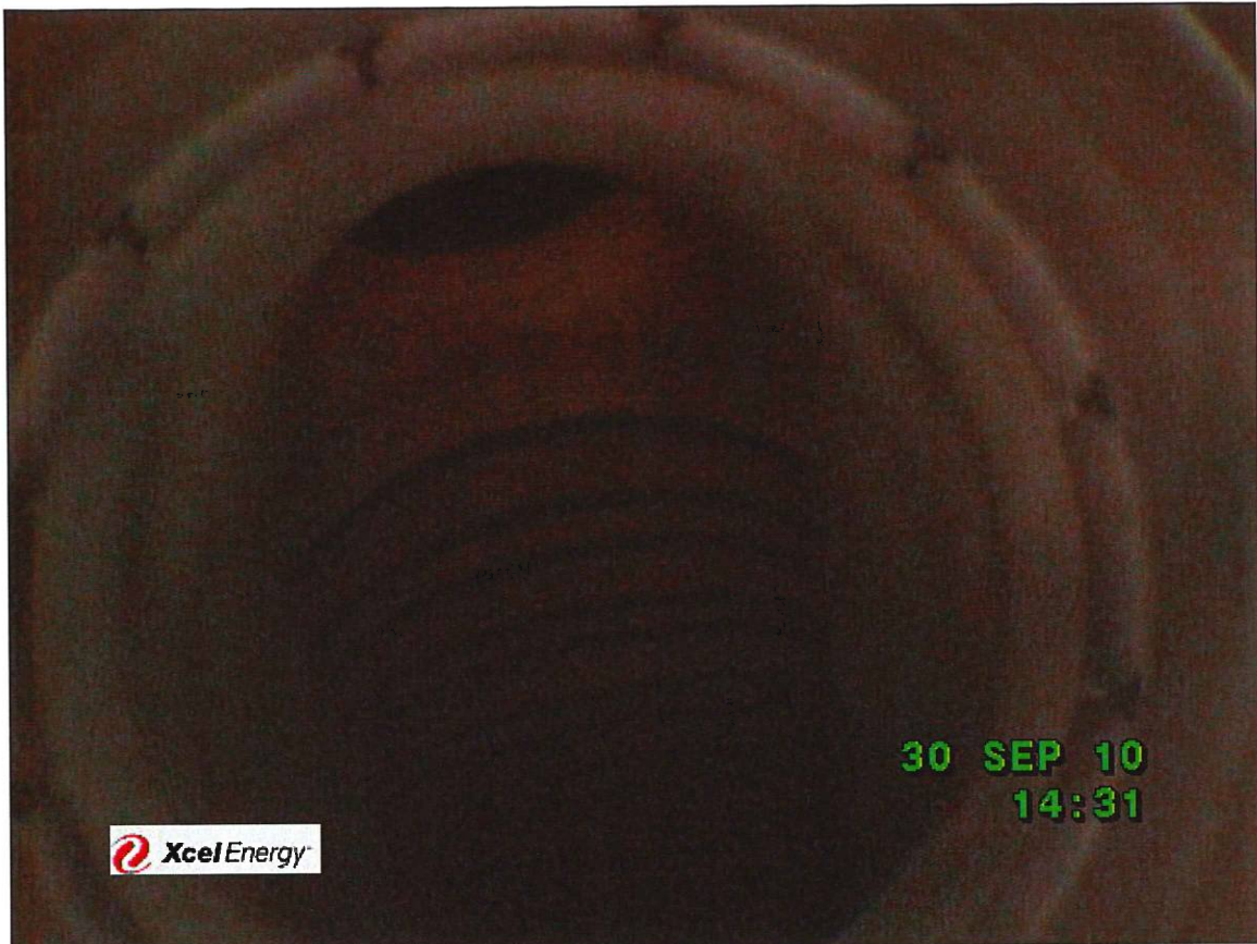
Unit 3, burner 3, view with borescope into transition area. No signs of cracking, or TBC coating loss at this point
