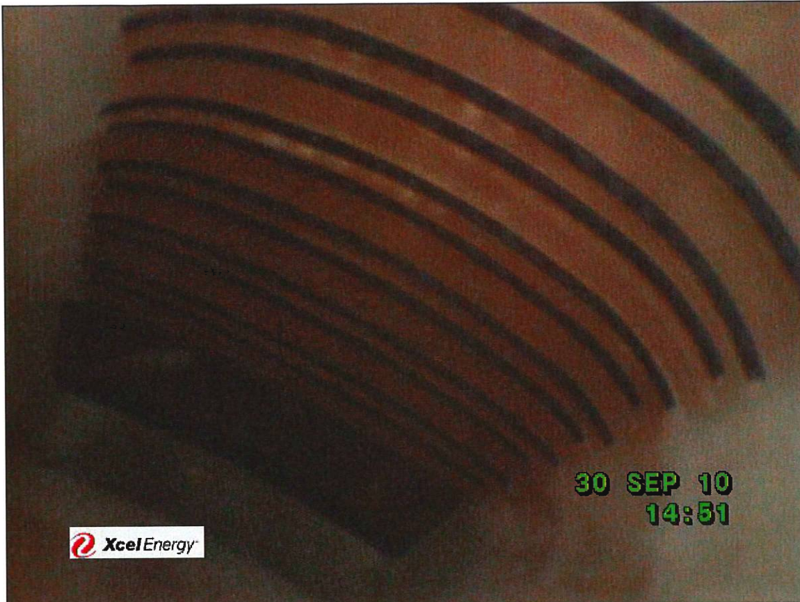
Borescope photo of transition outlet to row 1 vanes. General condition of the transition appears to be pretty good with no obvious signs of significant TBC coating loss.
