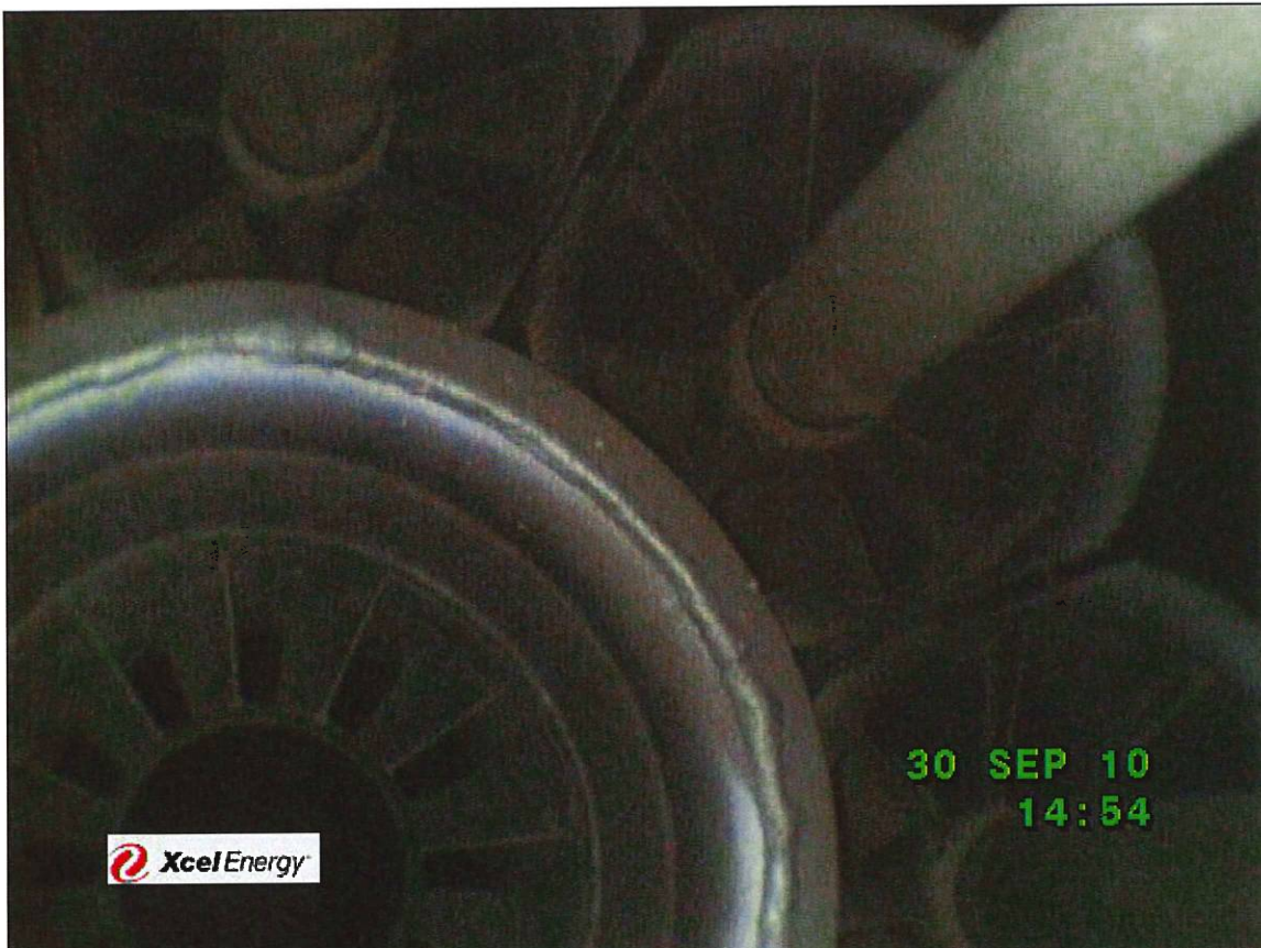
Pilot swirler and main fuel nozzles on burner #14 showing no significant problems.
