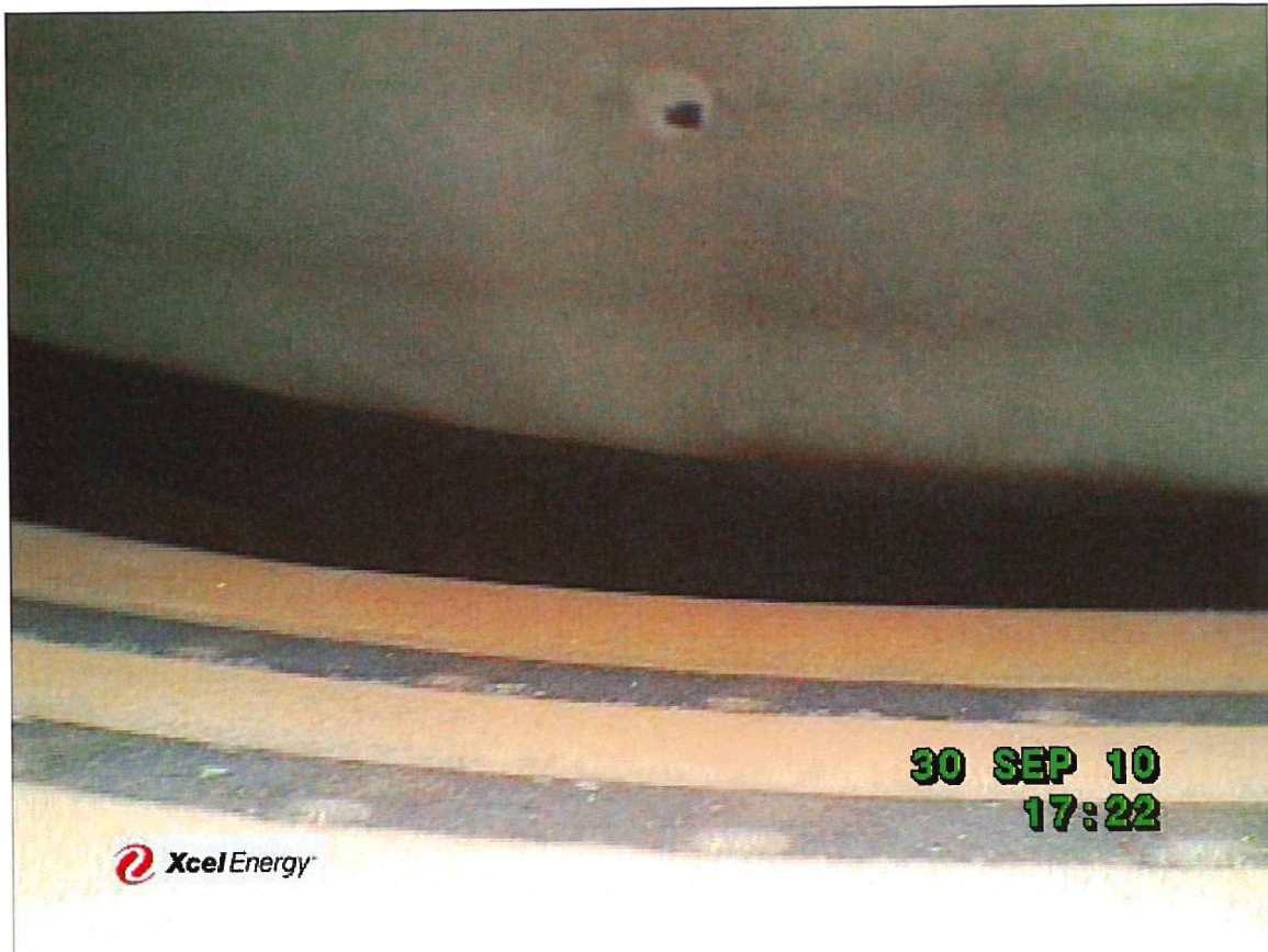
More minor TBC coating loss on #8 burner. This is believed to be typical of all, we just did not get sufficient detail on the transitions going through the pilot nozzle only.
