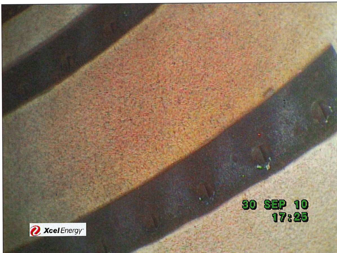
#8 burner transition cooling holes, no obvious signs of cracking or other distress.
