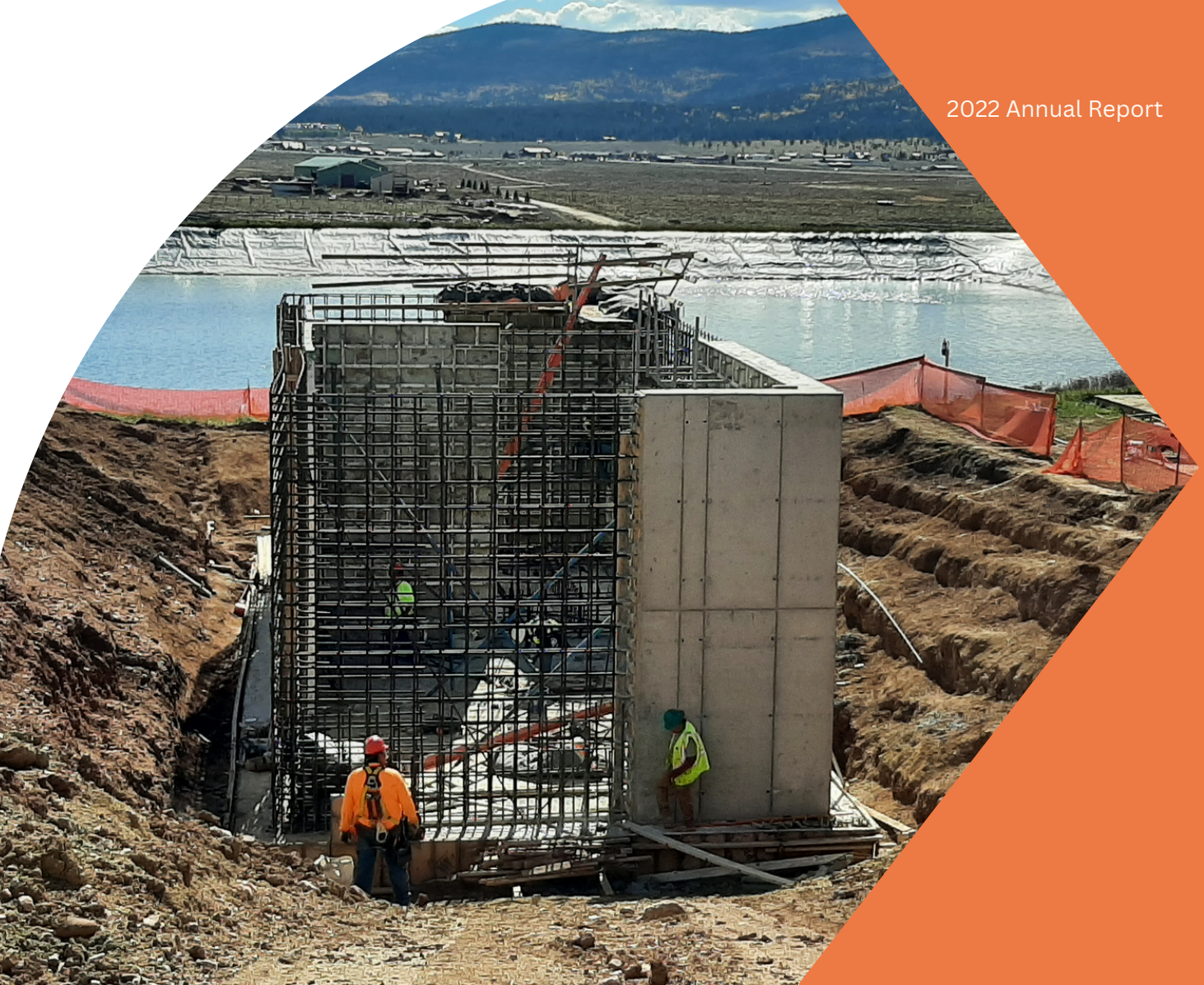
Angel Fire CWSRF 107 Post Equalization Aeration Basin
