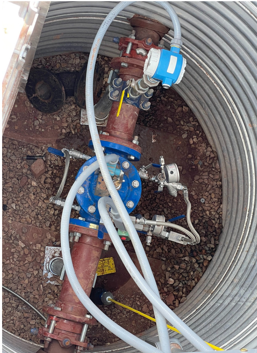
Well #3 solenoid control valve vault: Tijeras SAP 21-F2301-STB
