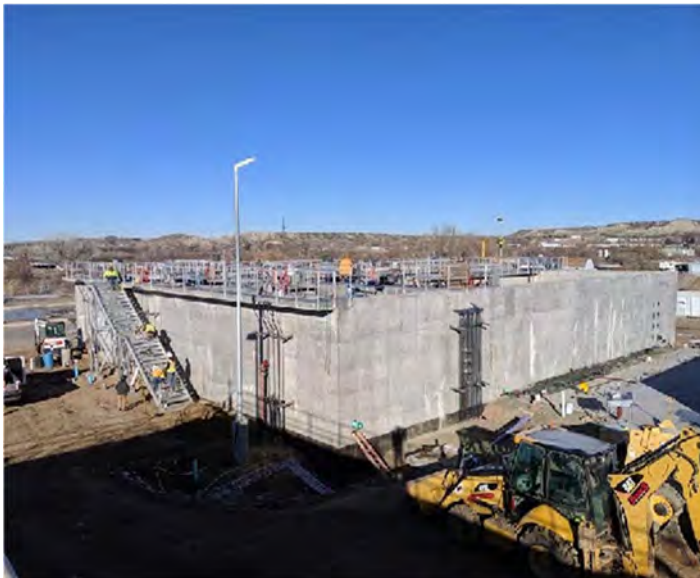
Sequencing Batch Reactor Digester
