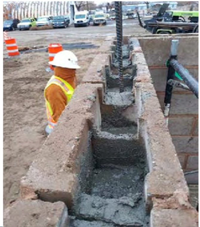
Grouting block cells and bond beam at Chemical Building CMU –City of Bloomfield
