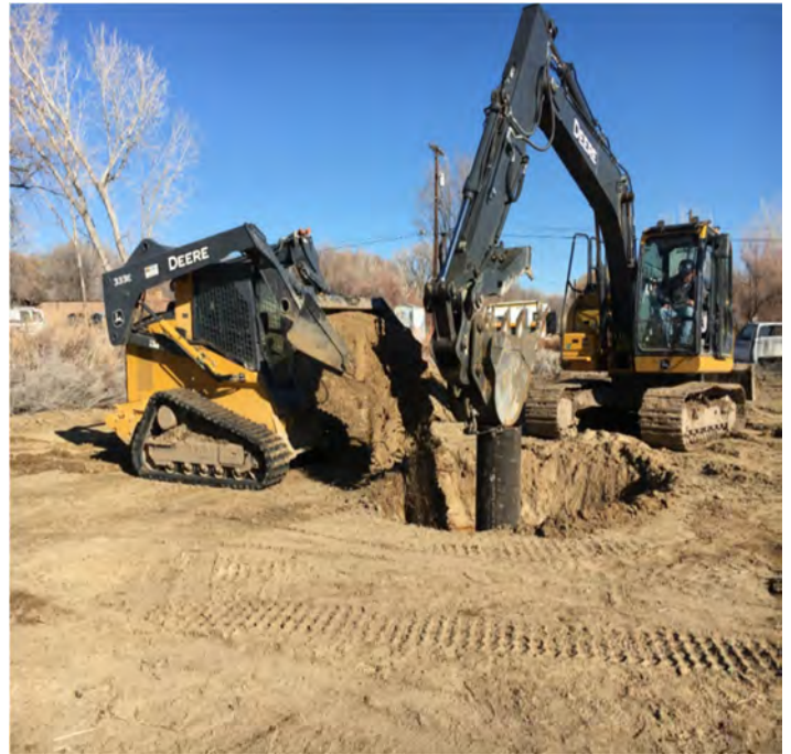
Drinking water wells for the Flora Vista Mutual Domestic Water Consumers Association
