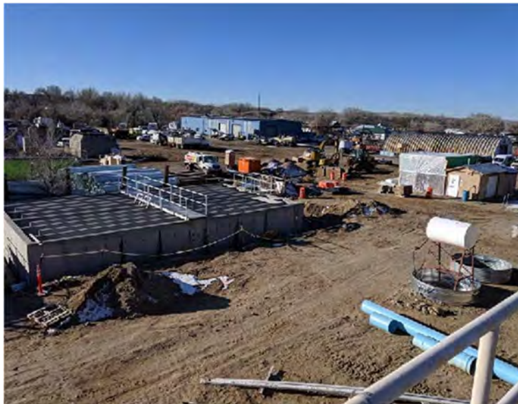
City of Bloomfield-Chlorine Contact Chamber
