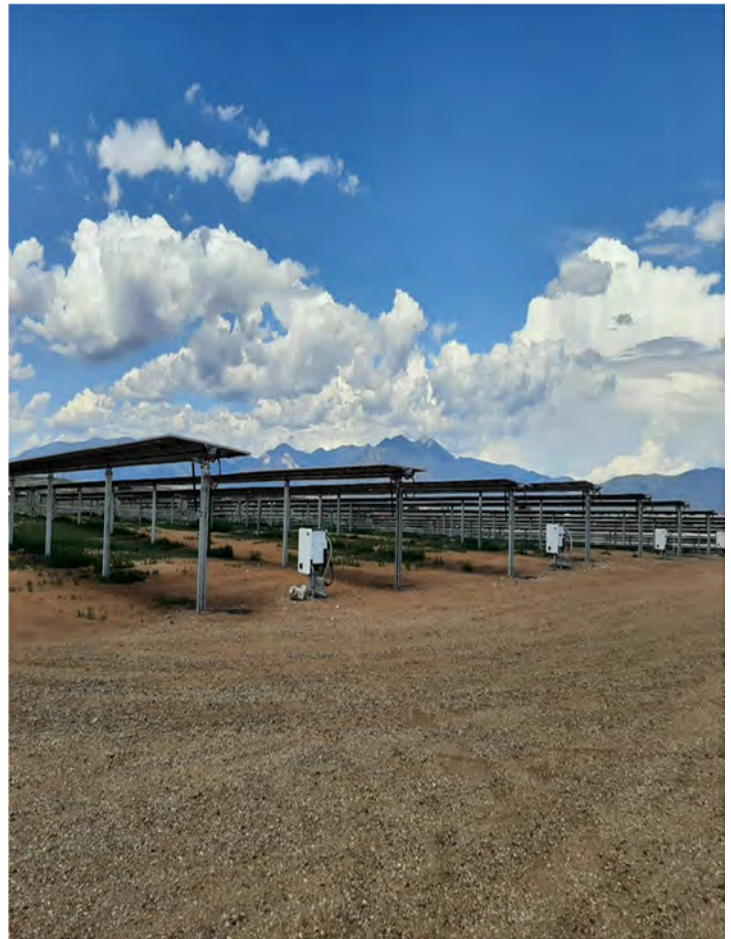
Town of Taos Wastewater Treatment Plant Solar Array
