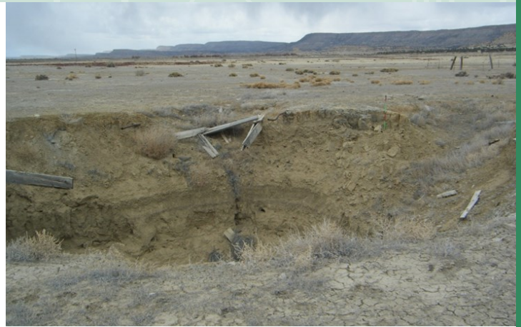
A large sink hole at a neglected AUM site in New Mexico. Neglected AUM sites may pose a physical danger to New Mexicans from pits, shafts (vertical entrances), adits (horizontal entrances), exposed waste rock, and other unstable mine structures.
