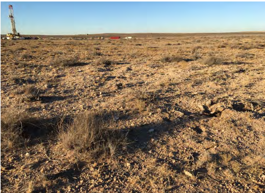
SP-6 View north from mapped outcrop of Qagp2 sand and gravel. Rig in background is drilling the Catalina 30 EH State 1H oil well, which is the location of the conductor pipe boring.
