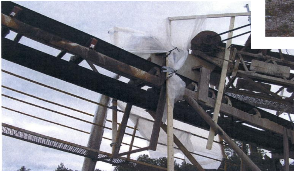
Figure 5. Conveyors, Hopper and Shroud
