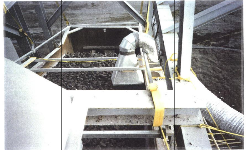
Photograph 6. Vibrating Screen, Track-Mounted Hood System, Structural Steel I Beam and Stone Flow Prevent Sampling in Upper 4 Feet of Vibrating Screen
