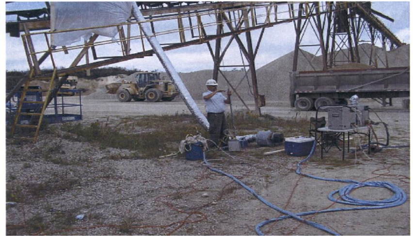
Figure 6. Sampling Equipment and Flexible Vent Line
