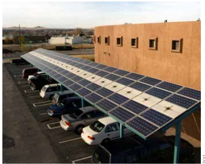
One of New Mexico's largest commercial solar PV installations can be found at the Indian Pueblo Cultural Center. This project is a successful example of how New Mexico could increase its renewable energy resources to reduce emissions and build resilience.
