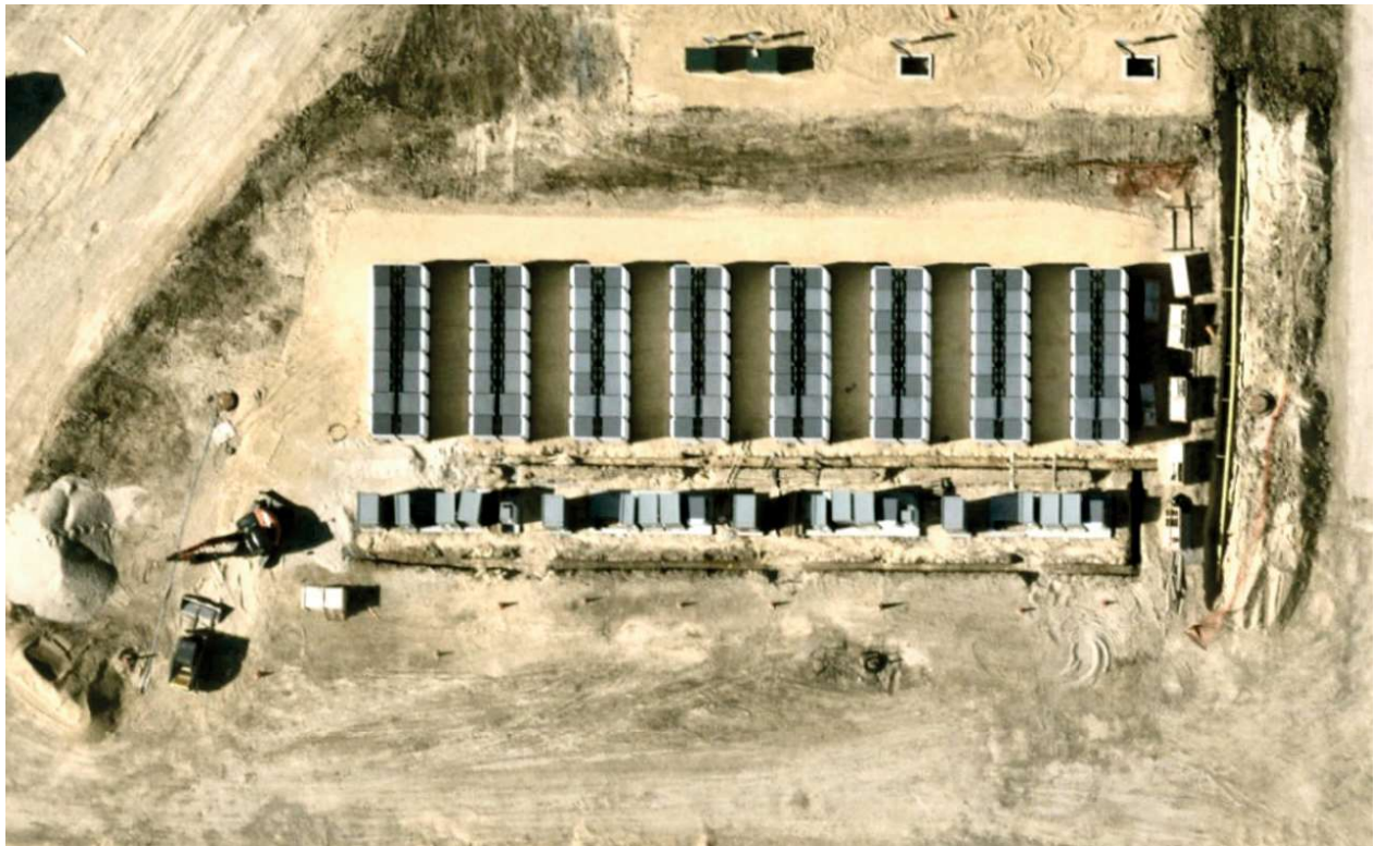
Bloom generators installed at CoreWeave's data center in Volo. Source: ArcGIS
