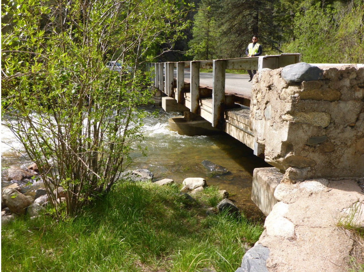
Figure 5. Picture of bridge #3926 (looking south) and the Rio Mora River located on NM 63 at the Mora Campground within San Miguel County, New Mexico.
