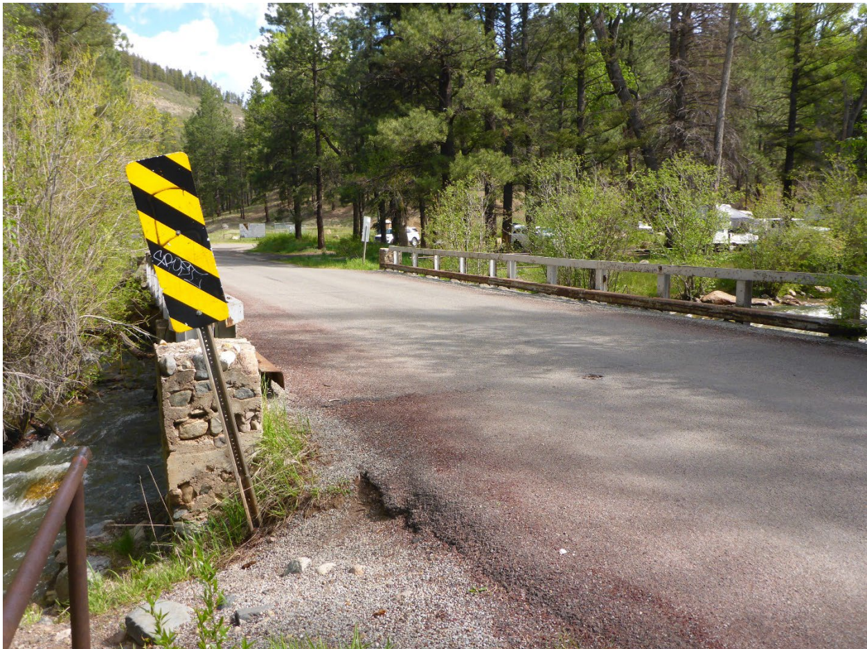
Figure 3. Picture of existing bridge #3926 (looking north) located on NM 63 at the Mora Campground within San Miguel County, New Mexico.
