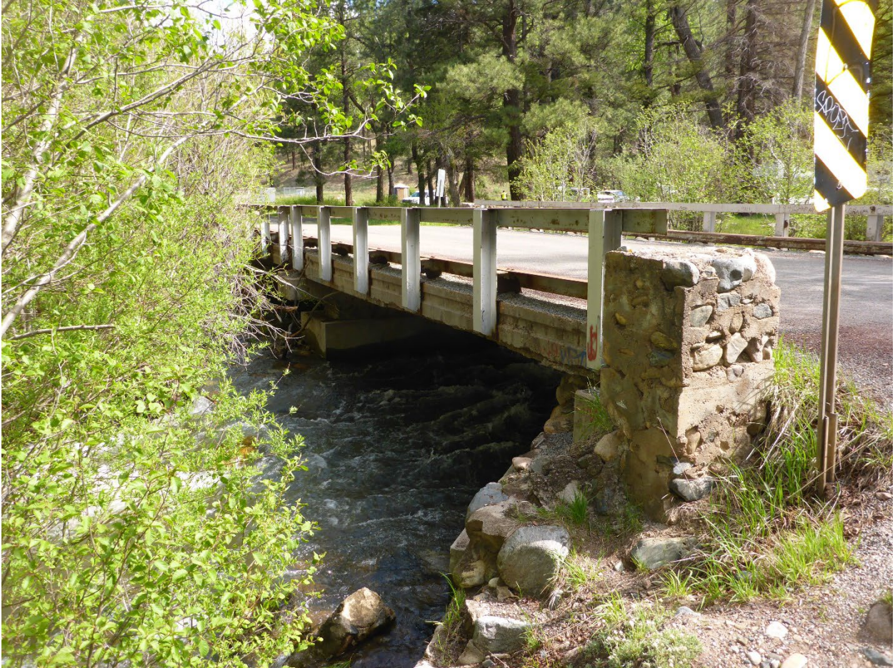
Figure 4. Picture of bridge #3926 (looking northeast) and the Rio Mora River located on NM 63 at the Mora Campground within San Miguel County, New Mexico.
