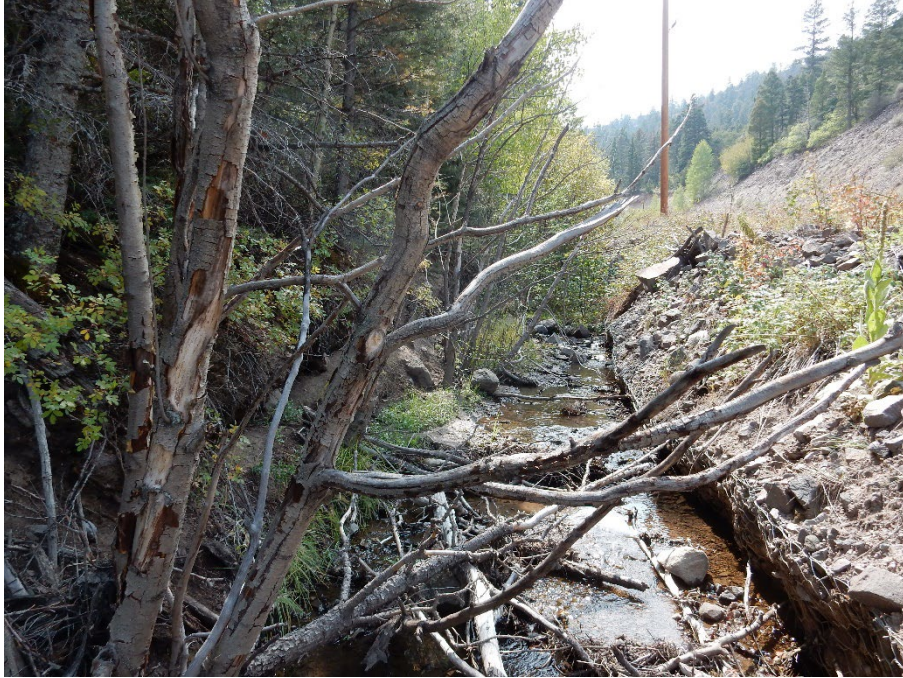
Figure 17. Example of Wetland Vegetation Zone Loss. The channel and adjacent wetland vegetation zone on Cordova Creek have been pushed over due to adjacent road placed in the narrow canyon. Road fill and revetment completely cover riverine wetlands on right side of channel and cause erosion of the left side of the channel and undercutting of vegetation.
