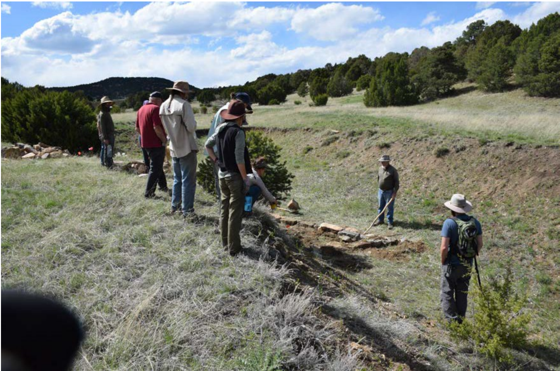
Figure 7. Participants are taught how to design and lead volunteers in installing restoration structures by Bill Zeedyk at Crew Leader Training at Rio Mora National Wildlife Refuge.
