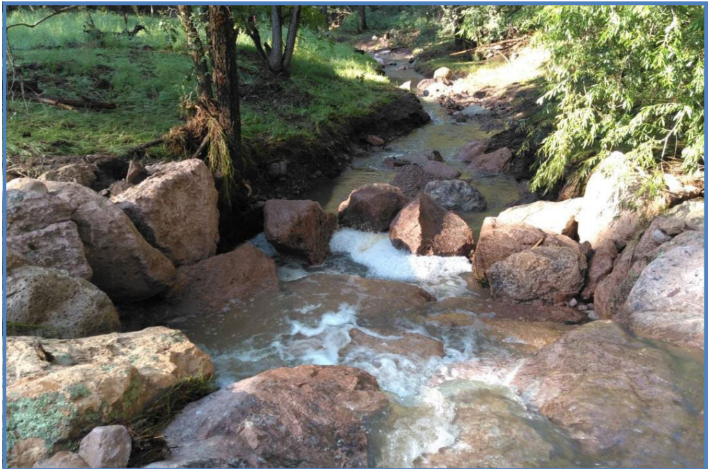
(Photo right): Cherry Creek in August 2022 after high flow events (view downstream). Sever- al boulders in this exam- ple grade control structure have moved downstream. This structure is visible from a different angle in Photo above.
