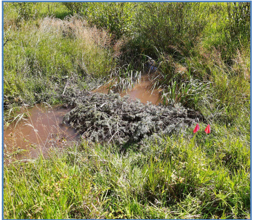
Instream structure intended to reinitiate stream floodplain connectivity by incorporating woody material within strategic locations of Rito Penas Negras.
