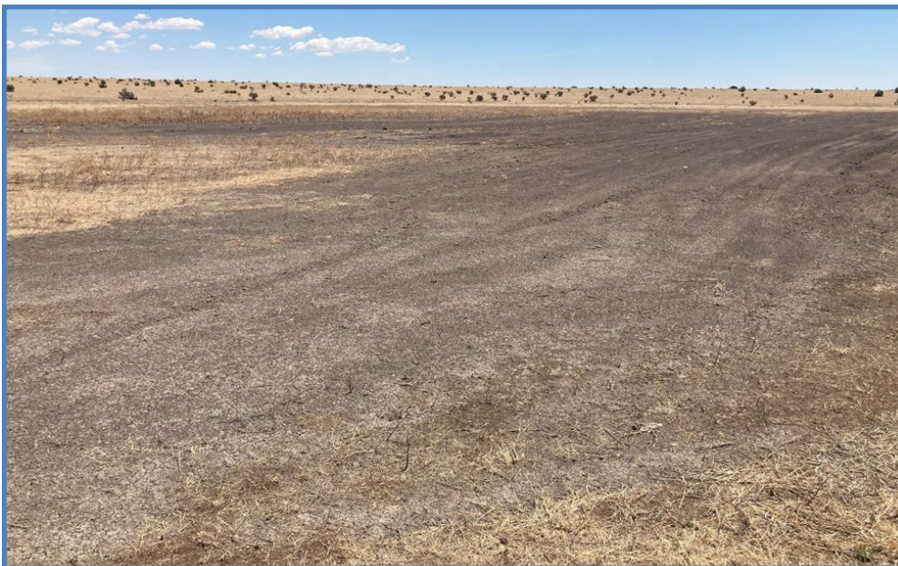
Post-restoration: The berm has been leveled out and the pit filled. Pho- to taken facing northeast. (6/10/22)
