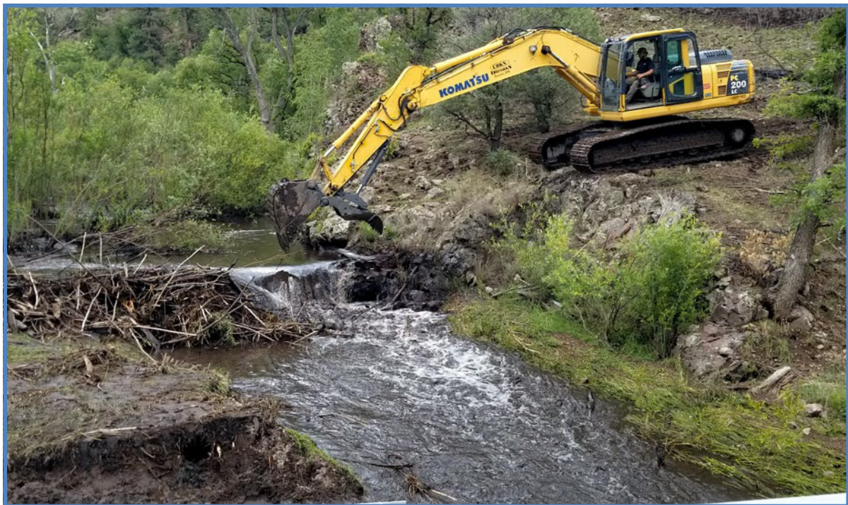
Removal of a beaver dam just upstream of Forest Road 150 bridge over Black Canyon Creek. This project was authorized under Section 404 Nationwide Permit 3 for maintenance activities.
