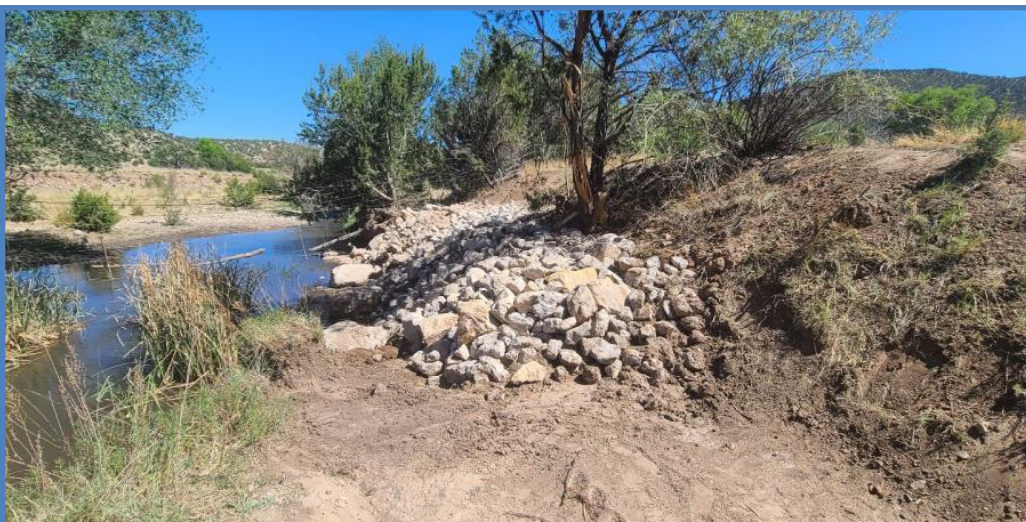
This post-project photo shows finished stream-bank stabilization structures and erosion control structures that the BLM Roswell Field Office installed along the Rio Bonito.
