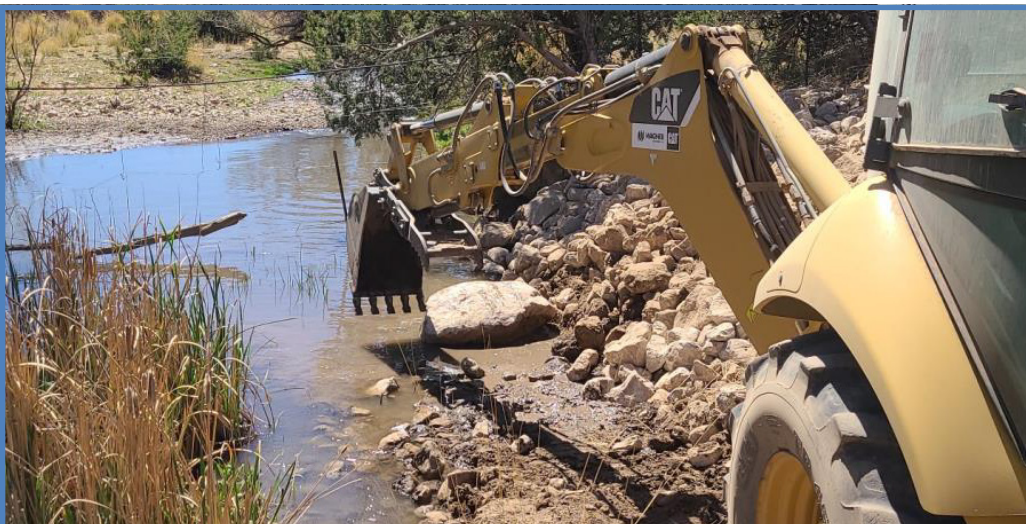
Installation of a single-stone bendway weir as part of a BLM Roswell Field Office project along the Rio Bonito.
