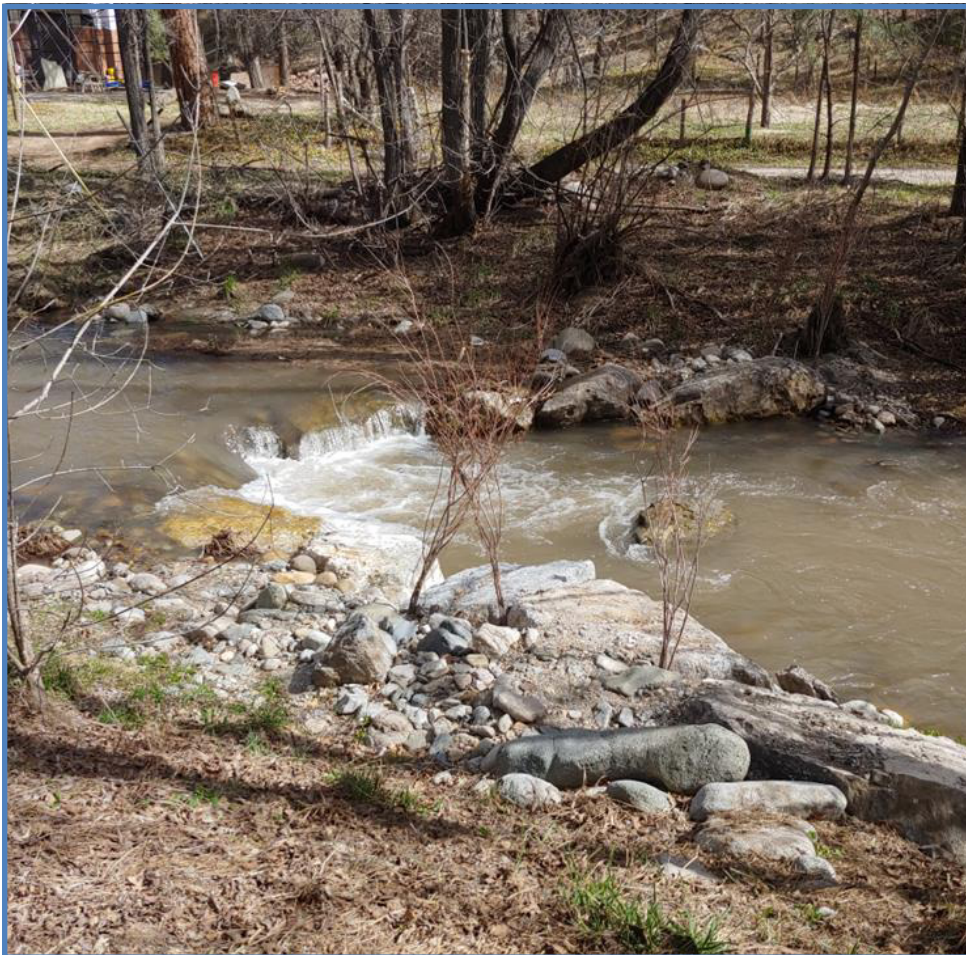
Photo left, Two Rivers Park Restoration Phase III – rock and woody debris convergence structure creating pool habitat.
