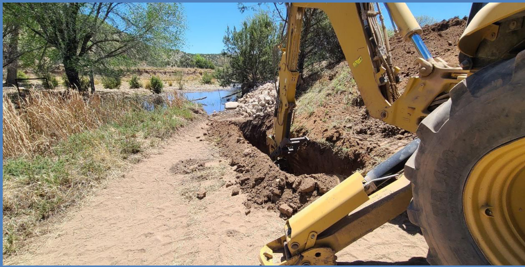
Installation of an erosion control tie-back dike as part of a BLM Roswell Field Office project along the Rio Bonito.
