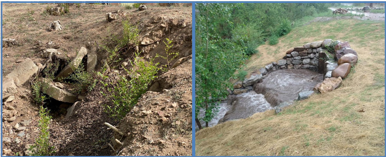
Before (left photo) and after (right photo). A Zuni bowl stormwater outlet drop structure was constructed in an urban area of Santa Fe to reduce E.coli and other pollutants in stormwater runoff before reaching the Santa Fe River. This is one example of a stormwater BMP that was designed for RSP project 20-M.
