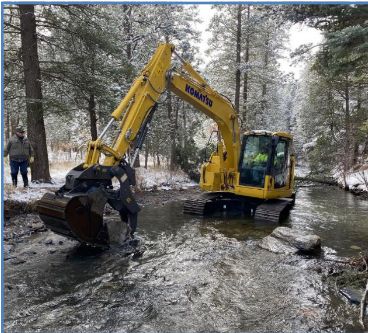
Photo left, Heavy equipment placing a habitat rock in the Cimarron River during a wintery day.
