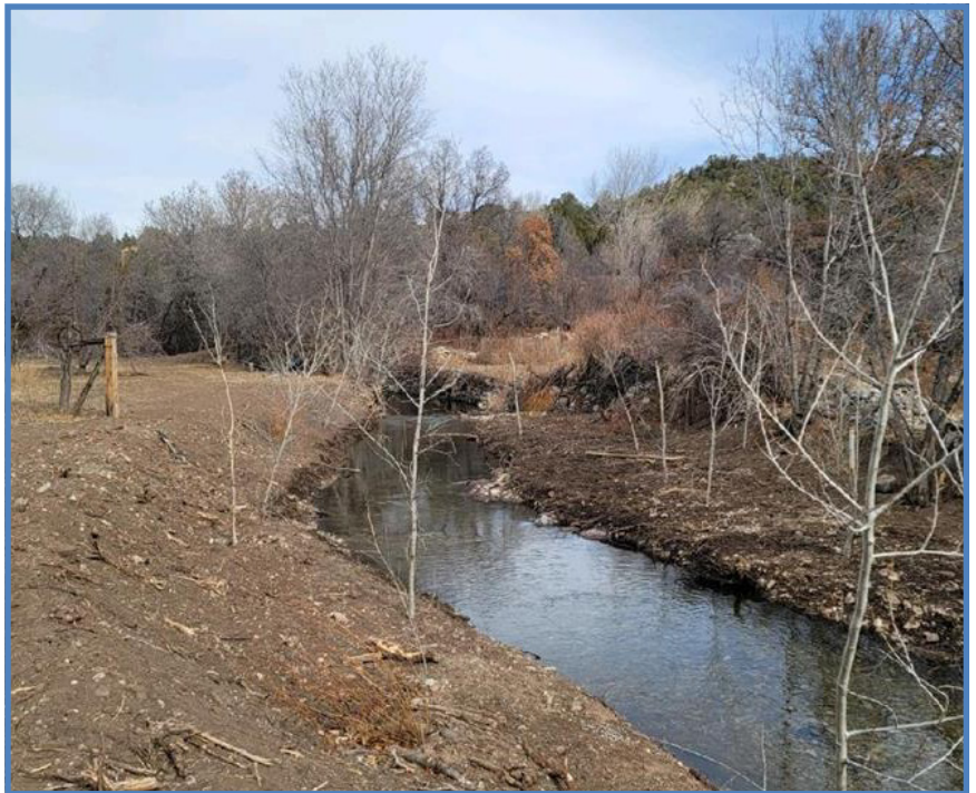
Photo above, Newly constructed bankfull bench planted with cottonwoods and willow. Bench allows for overbank flooding, reducing stream velocity and encourage sediment deposition.
