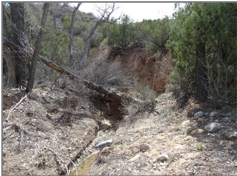
Wetland channel that eroded and became entrenched, leaving cottonwoods and willows high and dry and dying.
