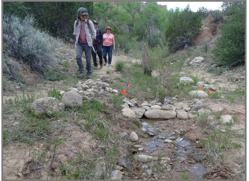
Workshop participants inspect their work at the end of the day building one-rock-dams and wicker weirs in the Labyrinth Spring canyon.
