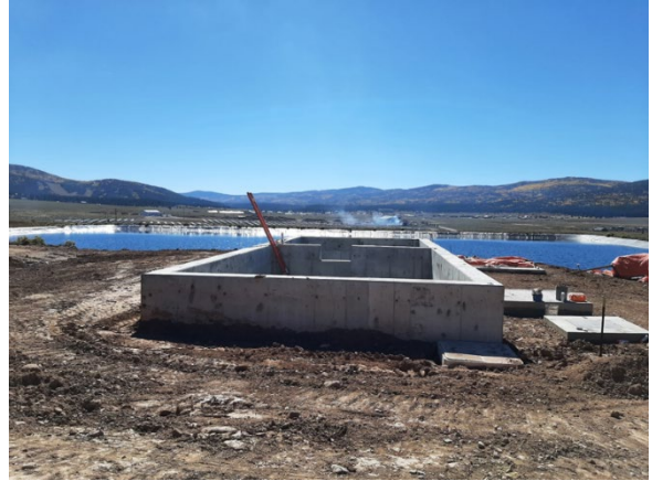
Village of Angel Fire CWSRF 107 New Post-Equalization / Post-Aeration Basin.
