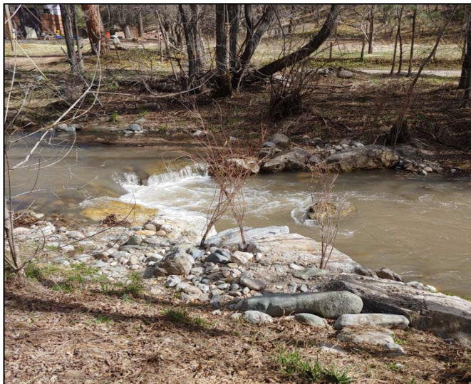
Two Rivers Park Restoration Phase III, RSP project in Ruidoso, NM, showing rock and woody debris convergence structure creating pool habitat on Rio Ruidoso.
