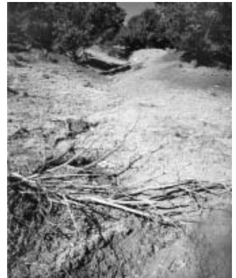
Rapidly eroding unprotected soil
