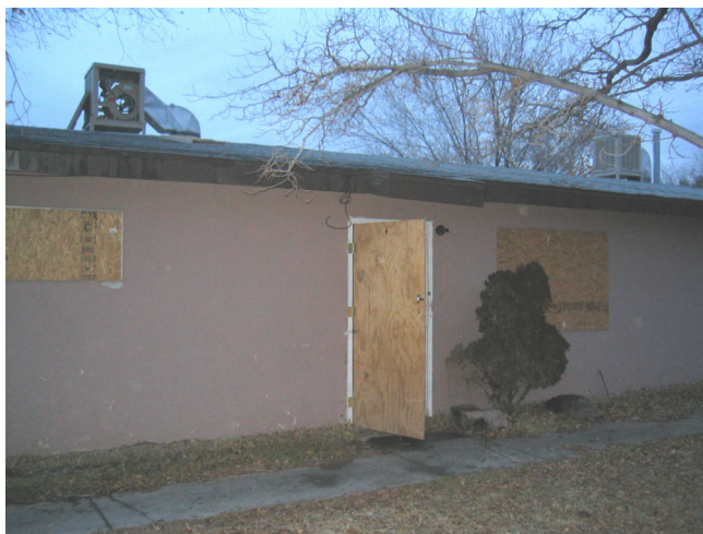
Figure 4. The site of cook #1 showing the closed windows and the door. Note the location of the evaporative cooler on the roof.
