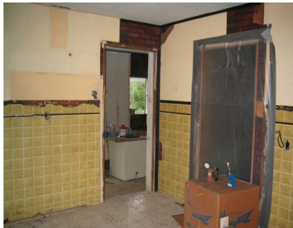
Figure 9. A picture from the adjacent room sampling area (third sampling area) into the cook area. Notice the door to the adjacent room has been sealed off.
