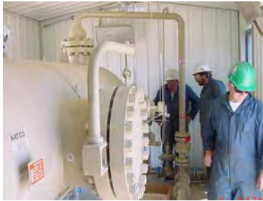
Three Phase Separator, Source: BP
