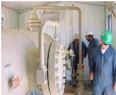
Portable Three Phase Separator, Source: BP
