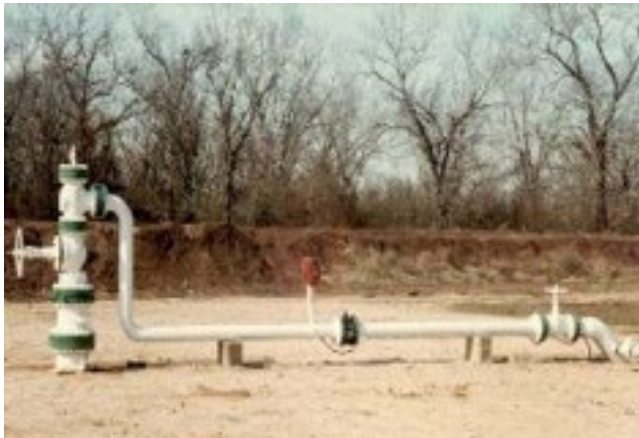
Currently, more than 90 percent of the produced water brought to the surface from the production of oil and gas is injected underground through Class II injection wells such as the one shown here to aid in future oil and gas production or for disposal.
