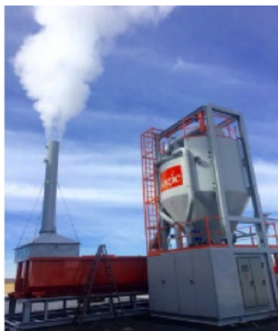
Figure 2-22: Evaporator Photo courtesy of Logic-ES
