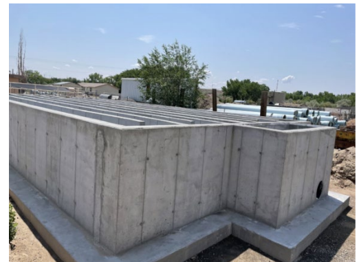
Chlorine Contact Chamber City of Bloomfield CWSRF 103
