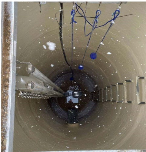
Return Pump Station City of Grants WSRF 077 (when snowing)
