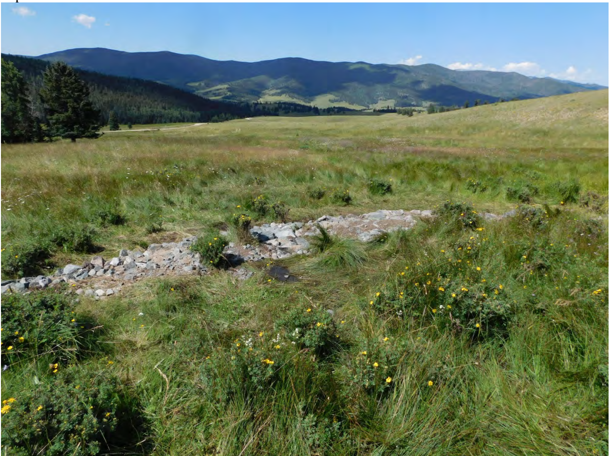
August 2019. A rock media luna was constructed to further spread from the flow splitter and lead out berm upvalley.
