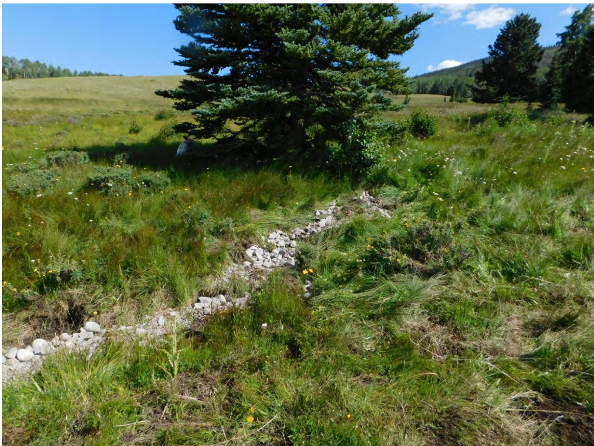
August 2019. Restoration treatment addressed an incised secondary channel through valley wetlands. High banks were collapsed and the new channel profile was armored with angular cobble (2019 NMDGF Funding).
