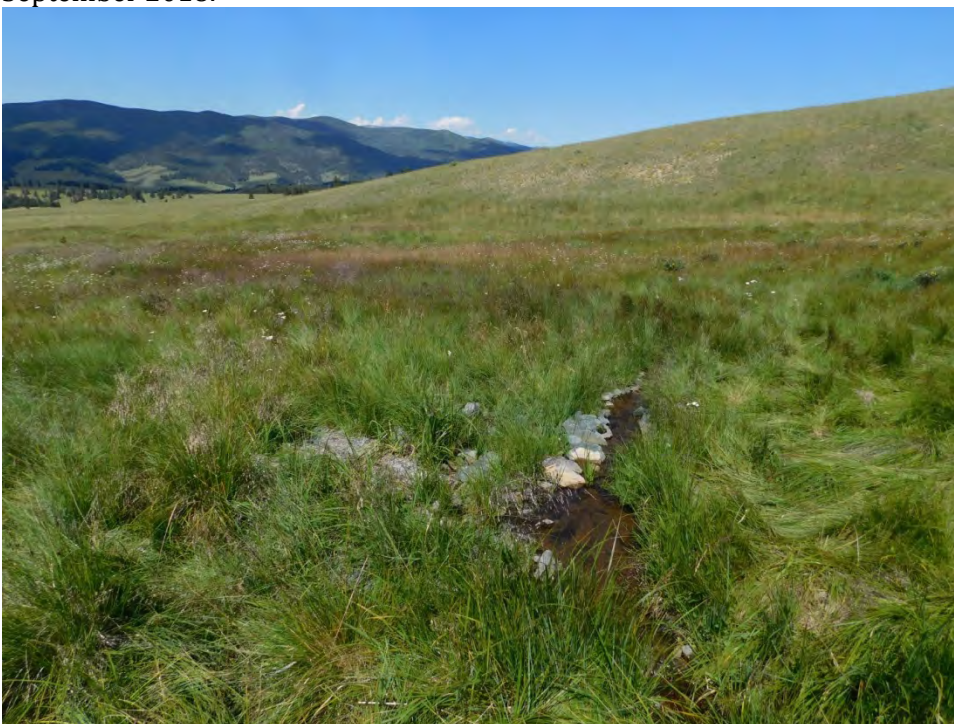
August 2019. A log mat flow splitter with rock armor was installed to move water to rewet a dried swale downslope at valley right.
