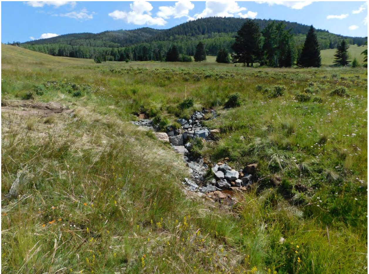
August 2019. Zuni bowl and large rock rundown constructed by Quivira volunteers and Reieneke Construction in 2019
