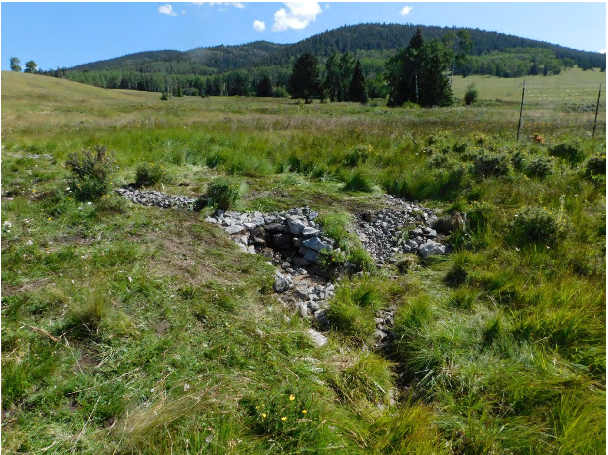
August 2019, Zuni Bowls and rock rundown to stabilize head-cutting and gully formation (2019 NMDGF Funding)
