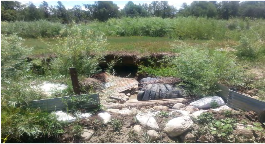
FIGURE 14 RIO NUTRIAS HEADGATE
