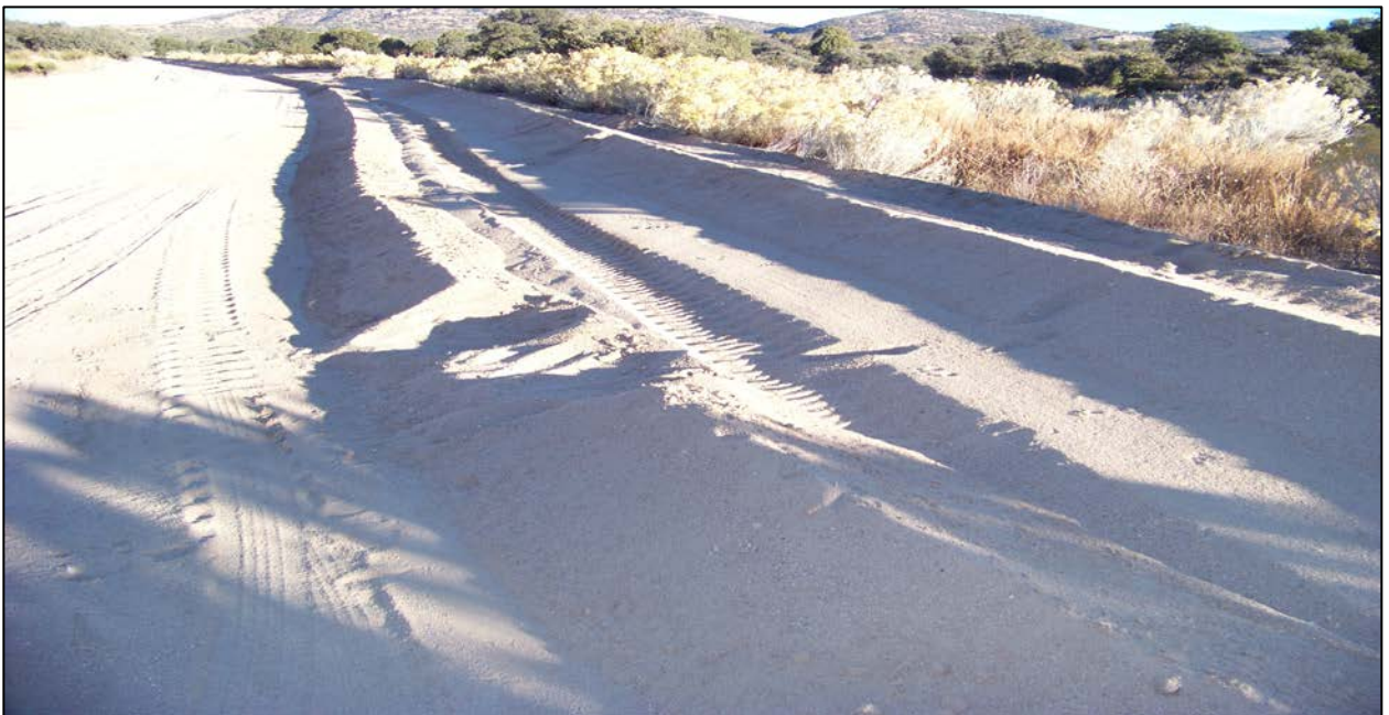
Photo 3. Major access road that now is a flood channel where large amounts of sediment are deposited and then bladed to the side to maintain the road.
