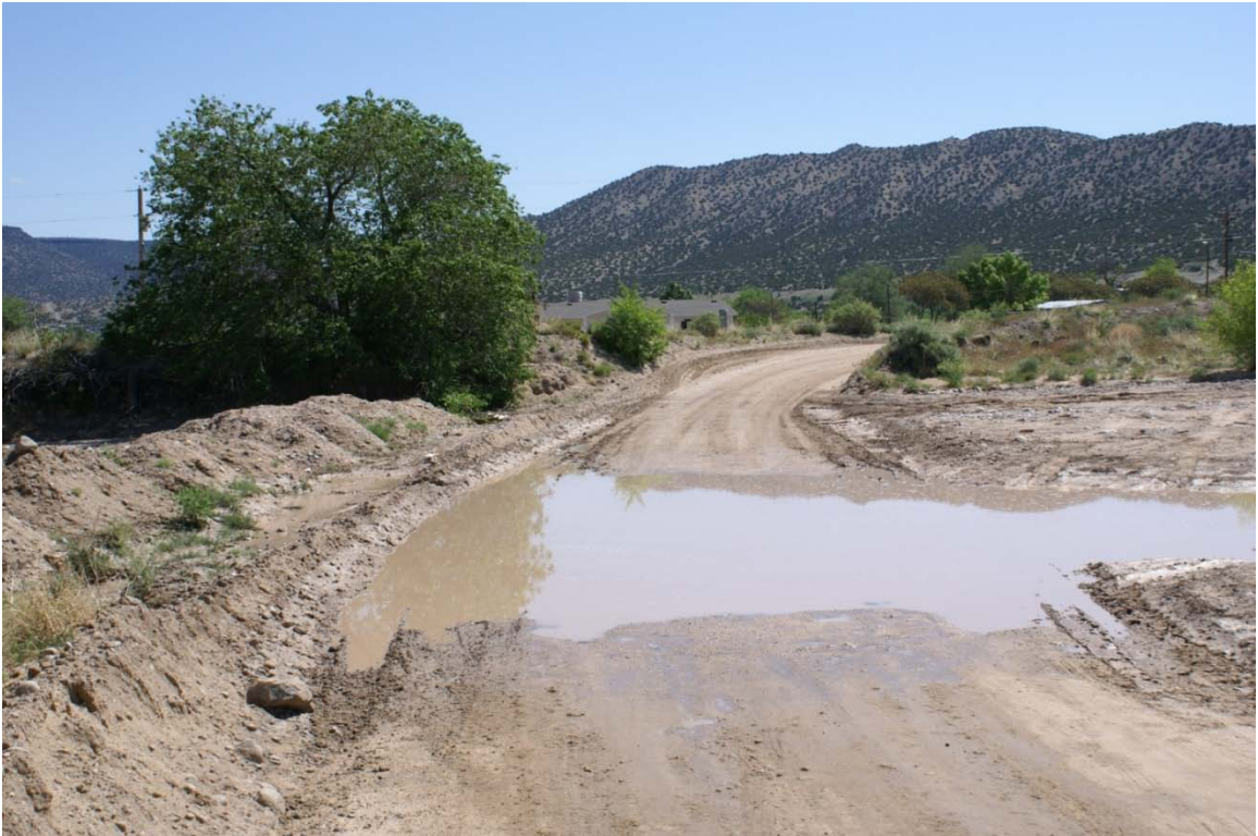
Figure 5 Flooded arroyo in Alcalde. (Johnston, 2007)
