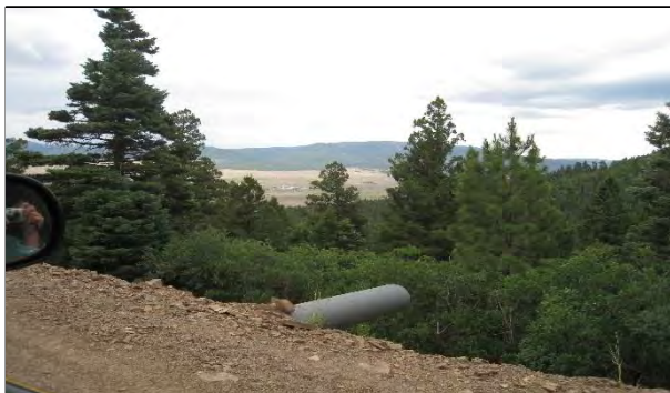
--Poorly placed culverts can accelerate erosion
