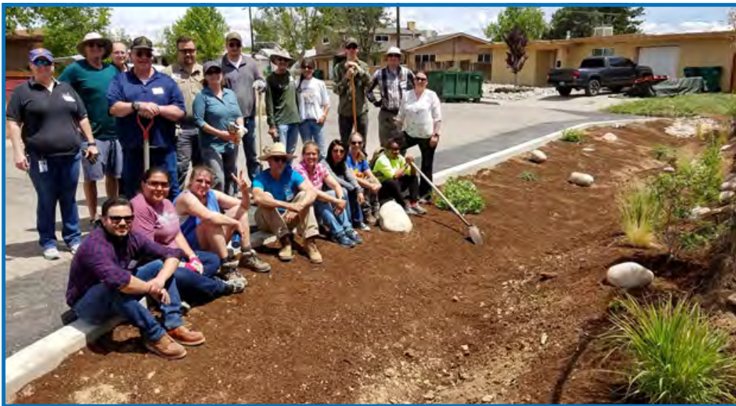
Workshop attendees pose for a photo after designing and constructing a demonstration project.
