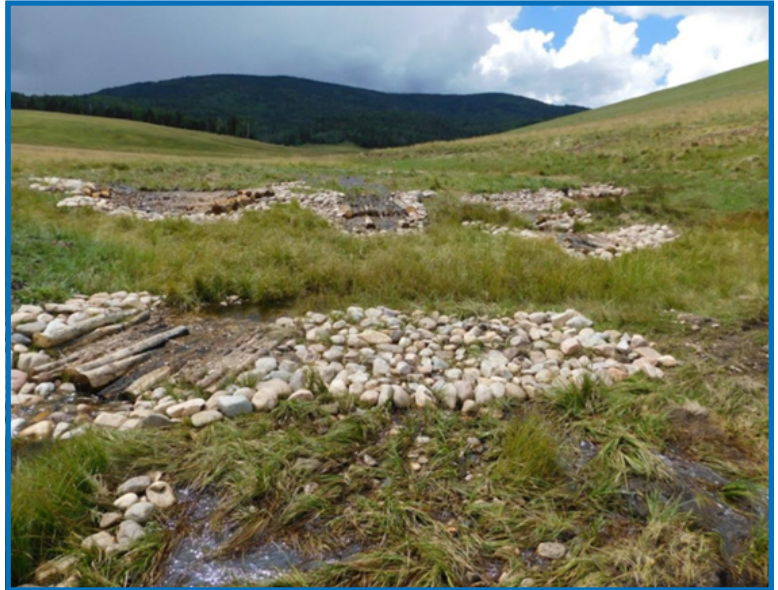
Foreman Creek with multiple log step-fall structures and one-rock dams to stabilize eroding wetlands.
