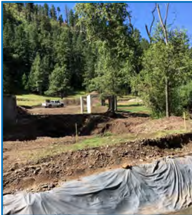
Re-route of new road and culvert to be installed along Bonito Creek.
