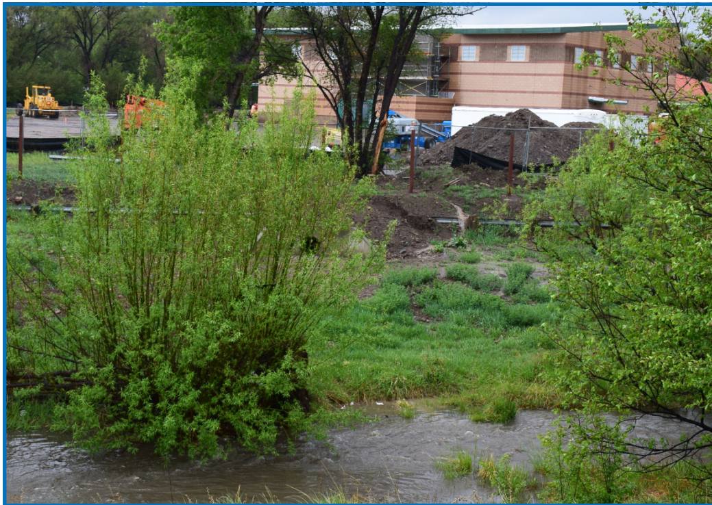
Polluted runoff from an improperly managed construction site carries sediment directly into the Gallinas River in Las Vegas, New Mexico. (photo by S. Styer)
