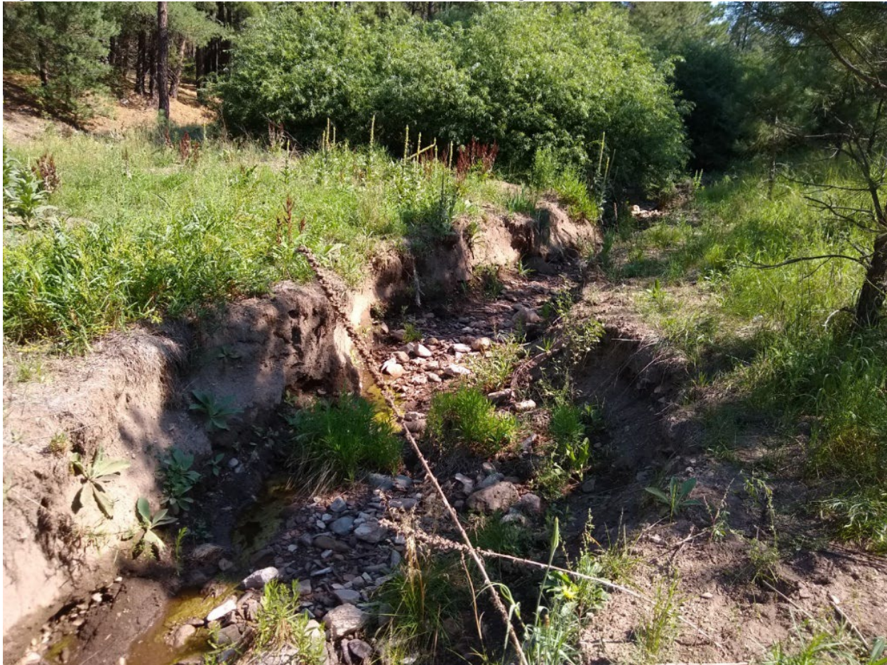
Figure 3. Soil and wetland loss due to channel widening (August 19, 2020)
