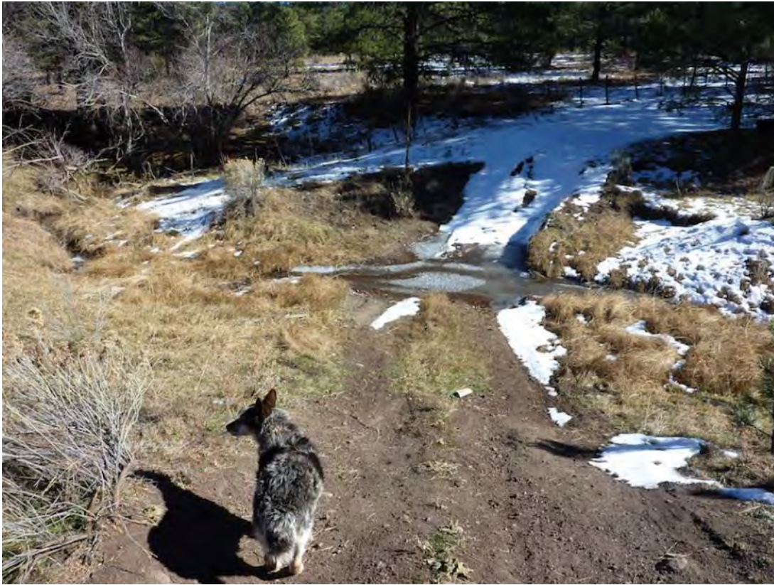
Figure 8. Two Track Road Crossing with Down Stream Eroding Banks
