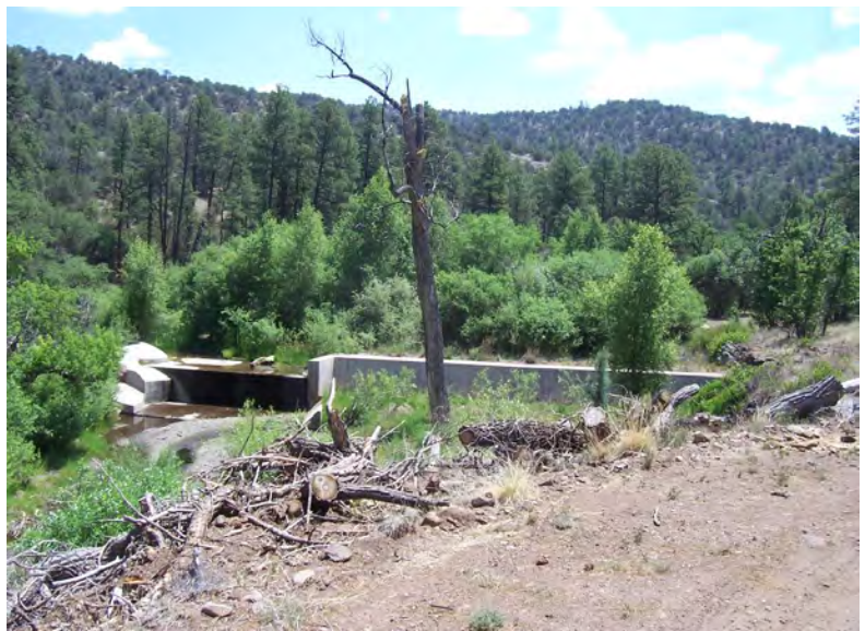
Figure 2. The fish barrier installed in Black Canyon Creek to prevent migration of non-native trout upstream.
