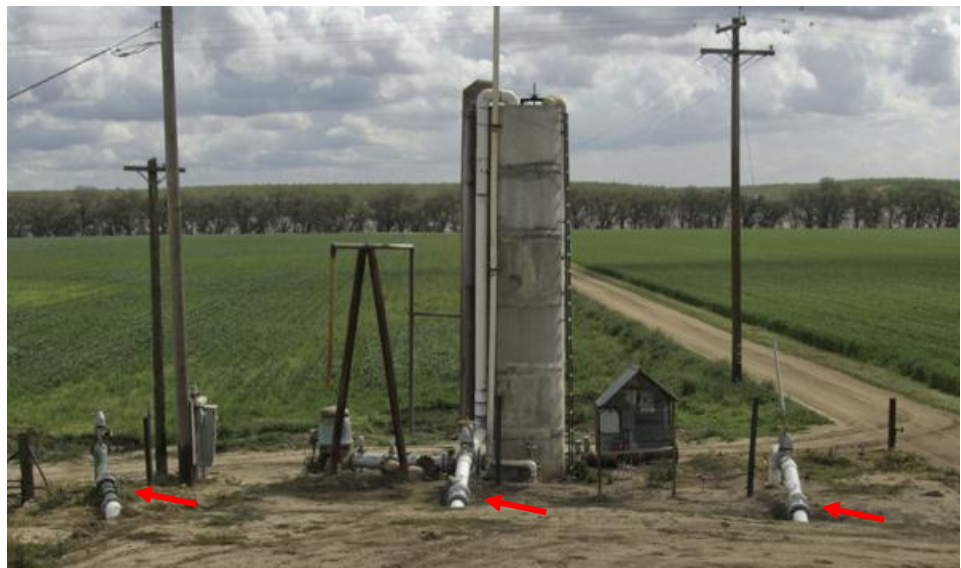
In this installation, separate metering runs allow lagoon water to be accurately applied on three locations simultaneously. A kiosk provides a lit, sheltered location to post target flow rates and record data.
