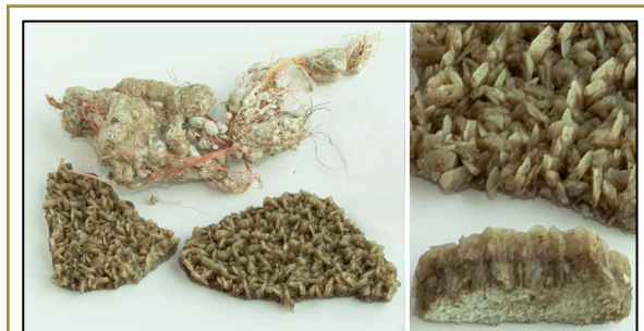
A crystalline deposit called struvite can form thick coatings on the inside of some lagoon pipelines. These will interfere with sensors that cannot be easily cleaned, and may be thick enough to change the diameter of the pipeline.
