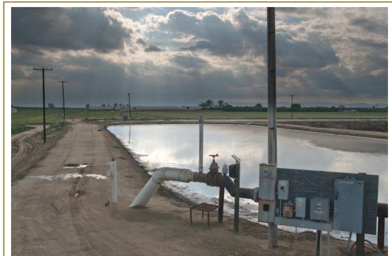
A flow meter on dairy lagoon discharge not only simplifies recordkeeping but enables the operator to accurately apply a predetermined rate of nutrients when used along with a flow control device such as a throttling valve.
