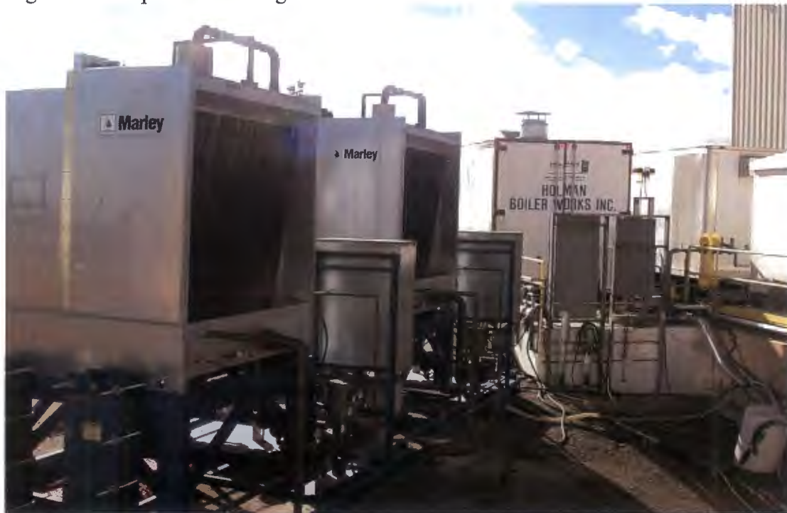
Figure 21. Evaporator Cooling Towers.
