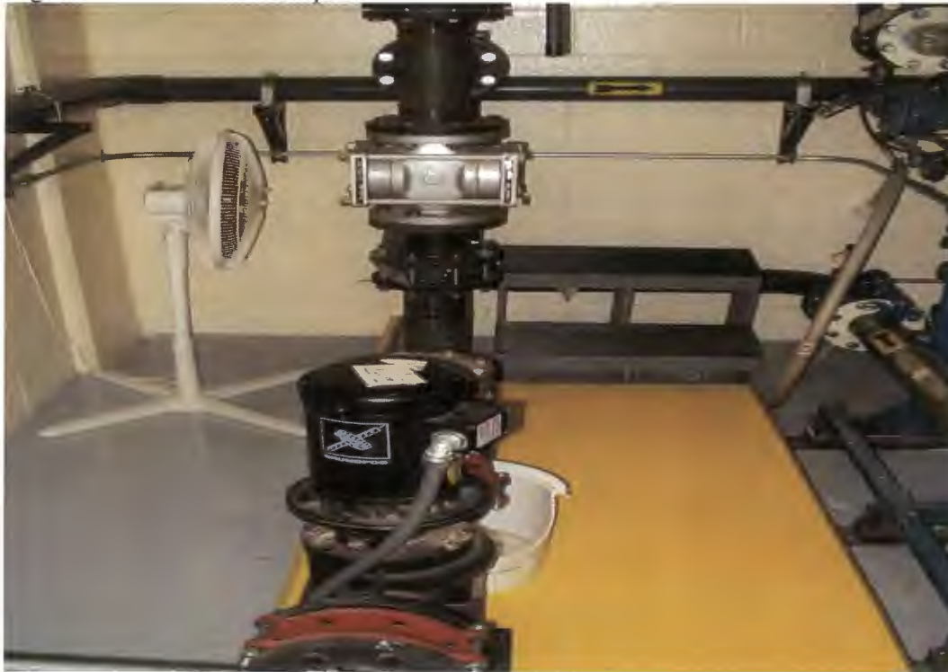
Figure 13. Motor and Pump.
