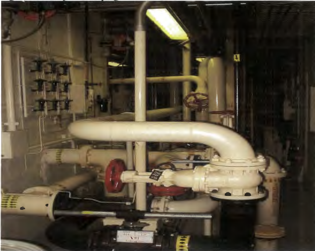
Figure 9. Gravity Filter Piping.
