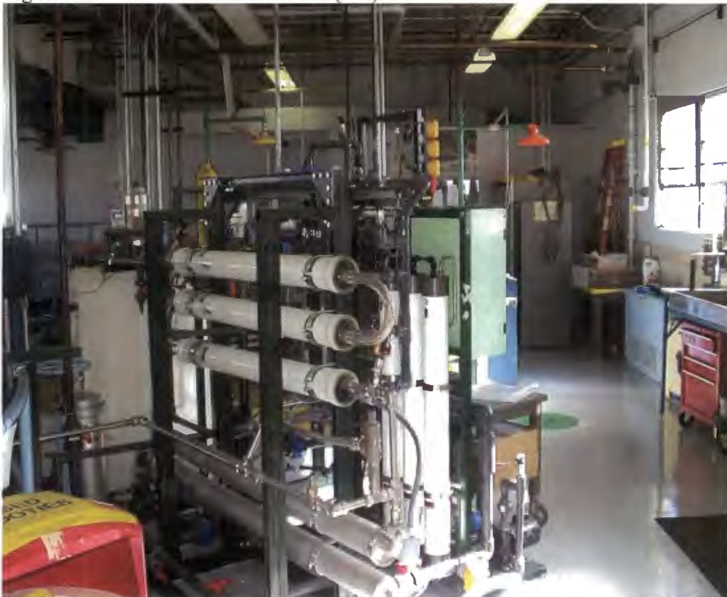
Figure 4. Seawater Reverse Osmosis (RO) Pilot Unit.
