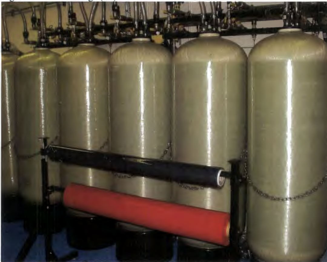
Figure 12. Ion Exchange (IX) Columns.
