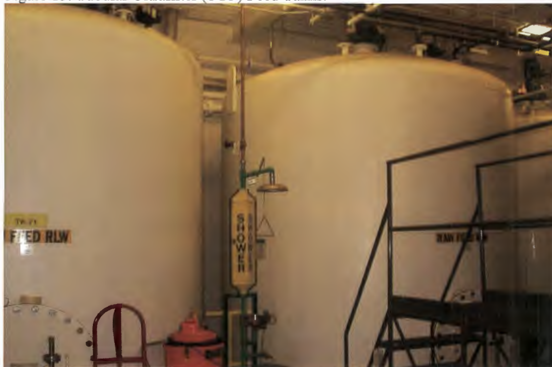
Figure 15. Tubular Ultrafilter (TUF) Feed Tanks.
