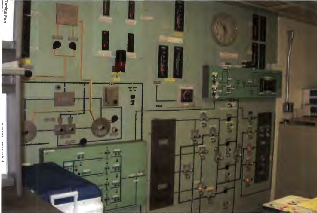
Figure 3. Older Control Panel.
