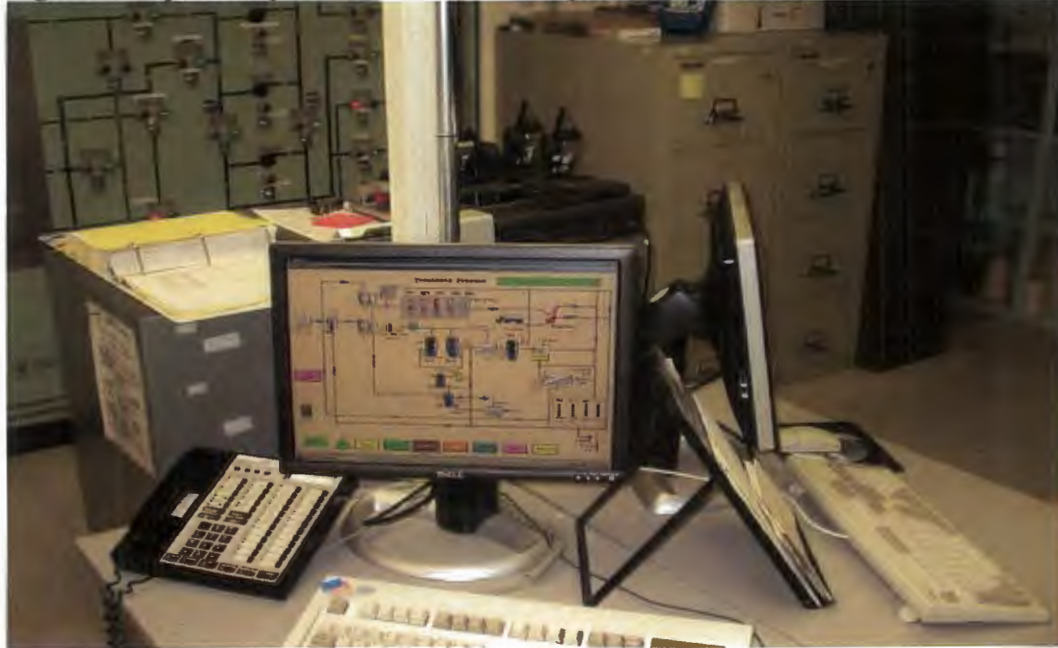
Figure 1. Supervisory Control and Data Acquisition (SCADA) Monitor.
