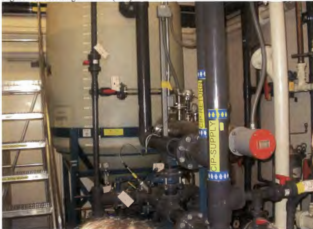
Figure 18. Cleaning-In-Place (CIP) Skid.
