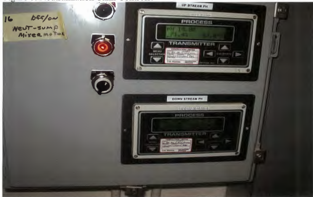
Figure 7. Neutralization Tank Controls.
