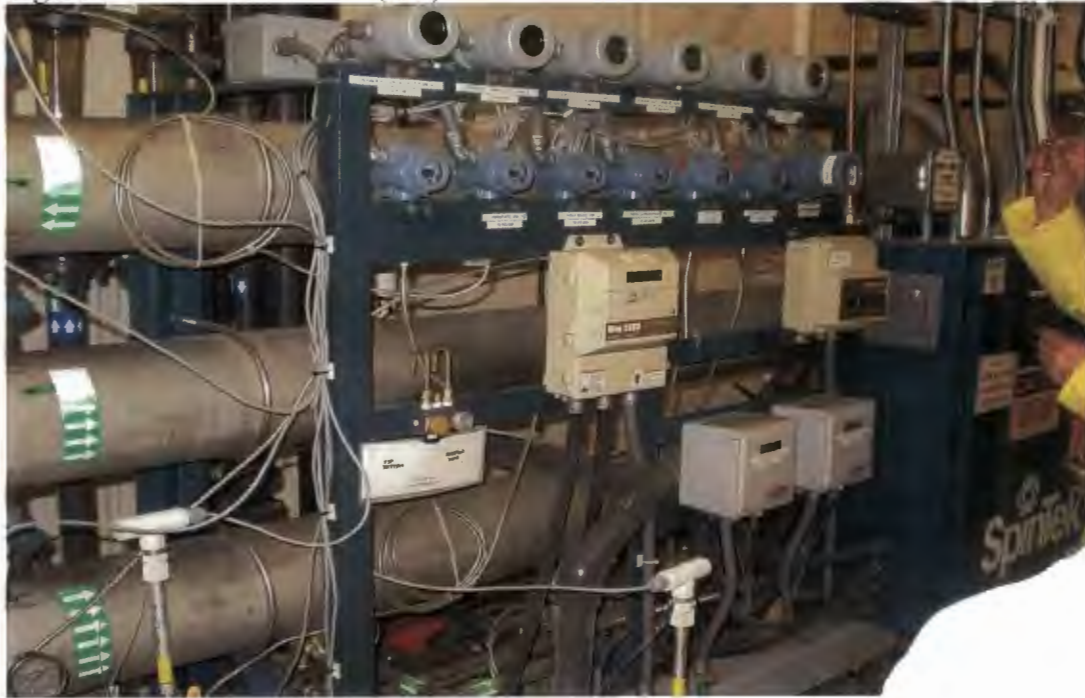
Figure 17. Reverse Osmosis (RO) Treatment Unit.
