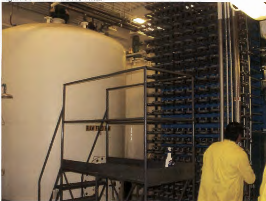
Figure 16. TUF and Feed Tanks.
