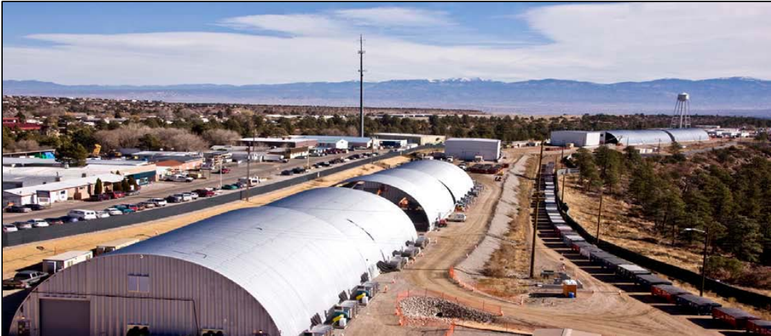
Overview photograph of enclosures and waste containers (right) at Material Disposal Area (MDA) B, looking east. (Photo courtesy of LANL.)
