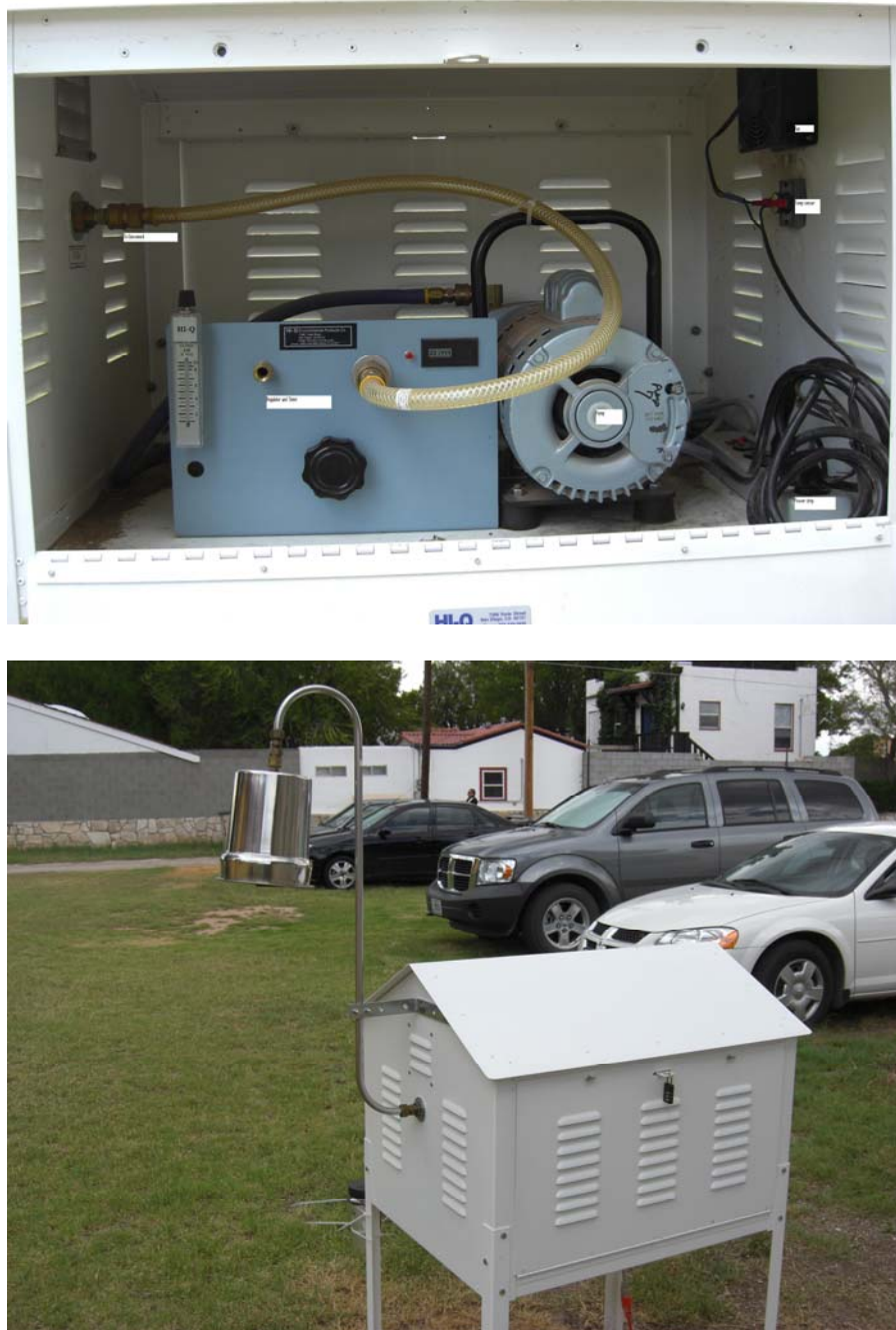
Figure SPL44-2. Inside and outside of a low-volume air monitoring station
