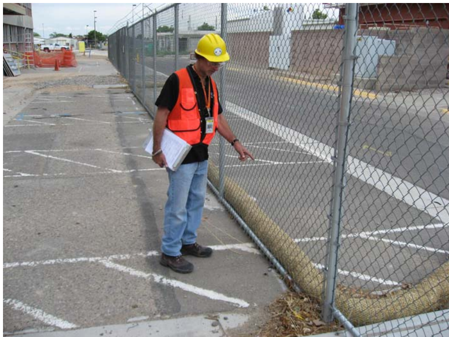
Figure SSW48-1. Staff discusses proper wattle installation at the Building 807 and 807A Decommission and Demolition Project at Sandia National Laboratories
