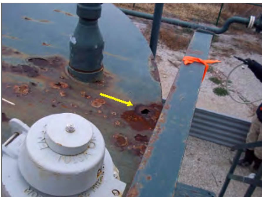
Figure 3.7-5. Hole in Tank Roof - Miscellaneous Emission Source
