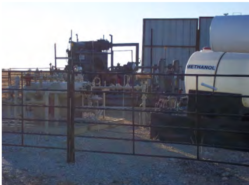
Figure 3.3-7. Site Documentation – Lift Compressor
