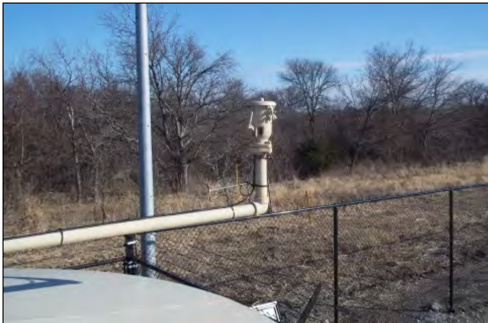
Figure 3.7-3. Storage Tank Vent
