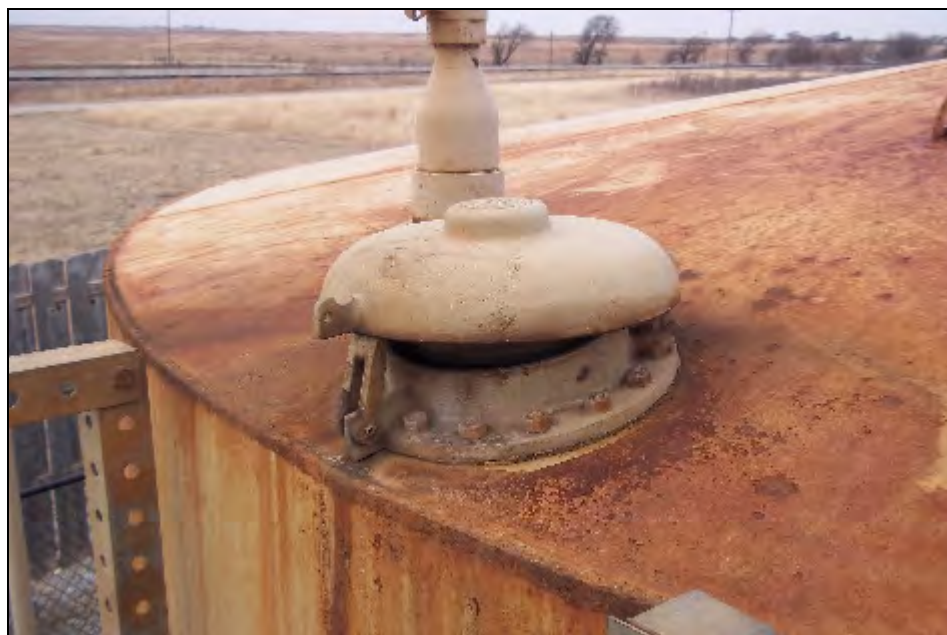
Figure 3.7-1. Thief Hatch Left Open
