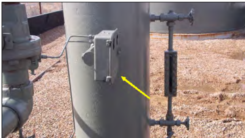
Figure 3.7-2. Pneumatic Valve Controller on Separator
