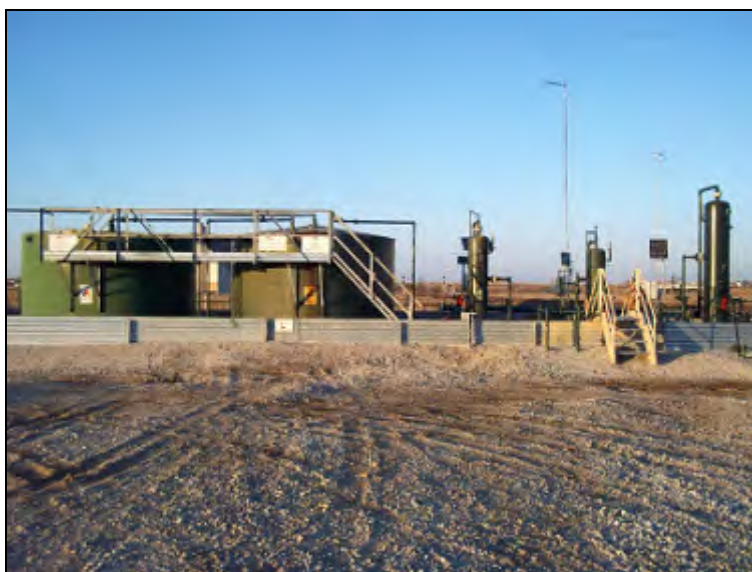
Figure 3.3-6. Site Documentation – Tanks and Separators
